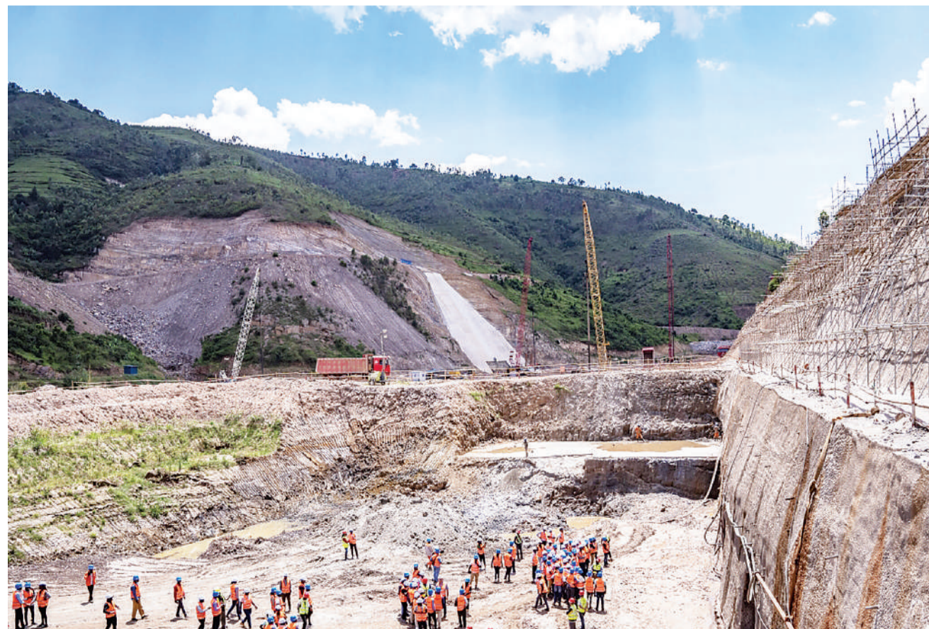
Engineers during a study tour at the ongoing construction activities of Nyabarongo Hydropower plant.
