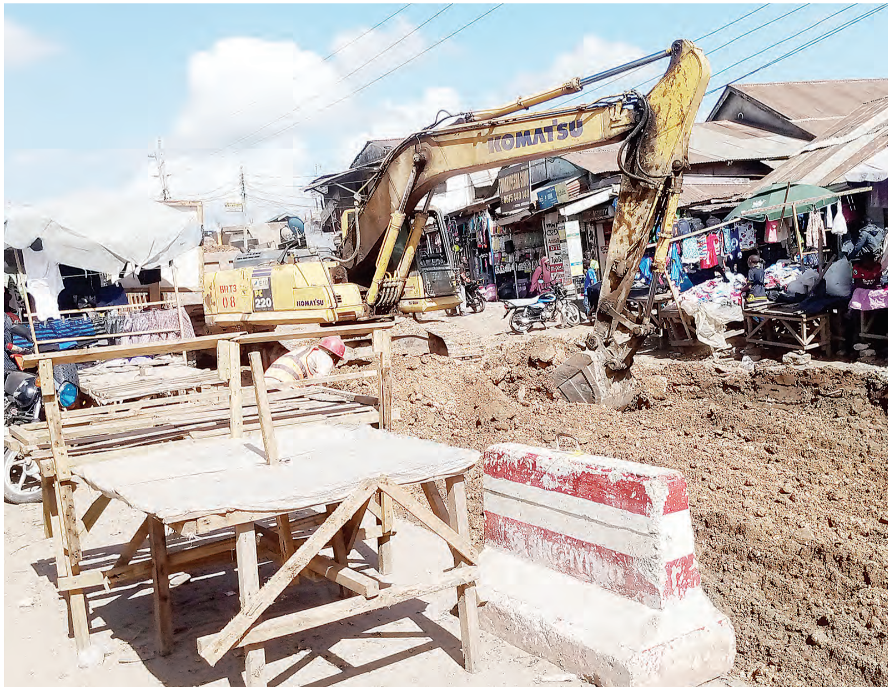
Construction of Dar es Salaam's rapid transit bus project infrastructure in progress along the Gongo la Mboto stretch of Nyerere Road yesterday. Photo: Correspondent Sabato Kasika
