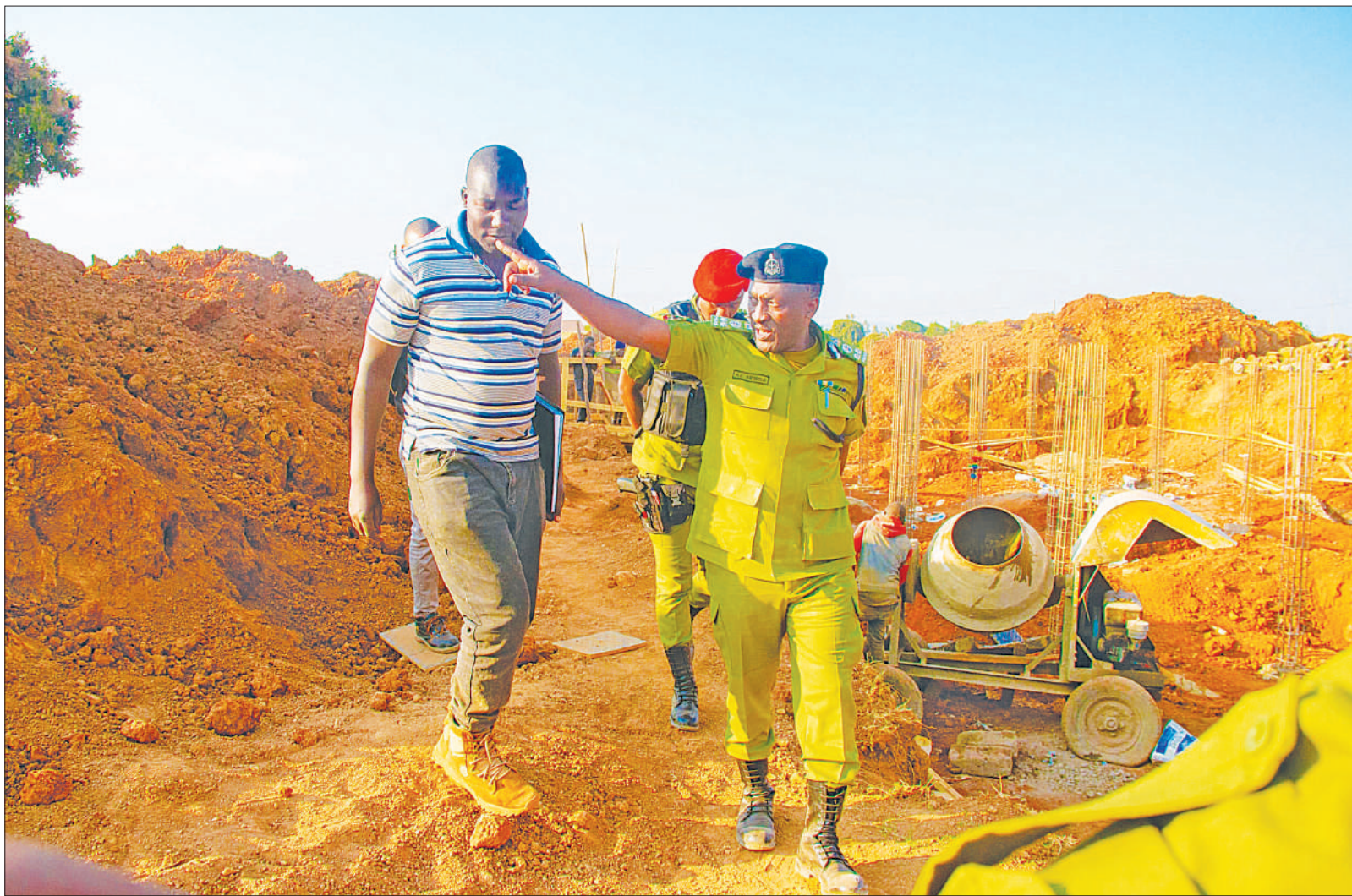
Augustino Senga, the Songwe regional police commander, inspects police post construction within gold mining area yesterday, to assess the security situation in the area. Photo: Correspondent Ibrahim Yassin
