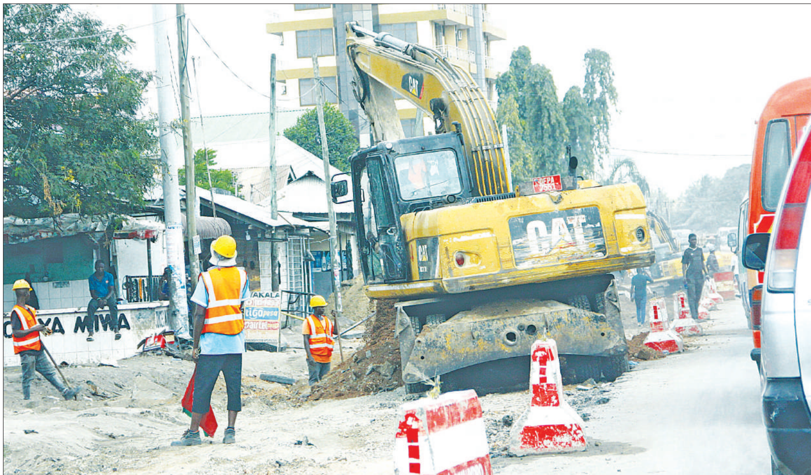
A caterpillar removes soil to harden the base during construction of a portion of the city Bus Rapid Transit routes at Ilala Bungoni yesterday. Photo: Correspondent Jumanne Juma
