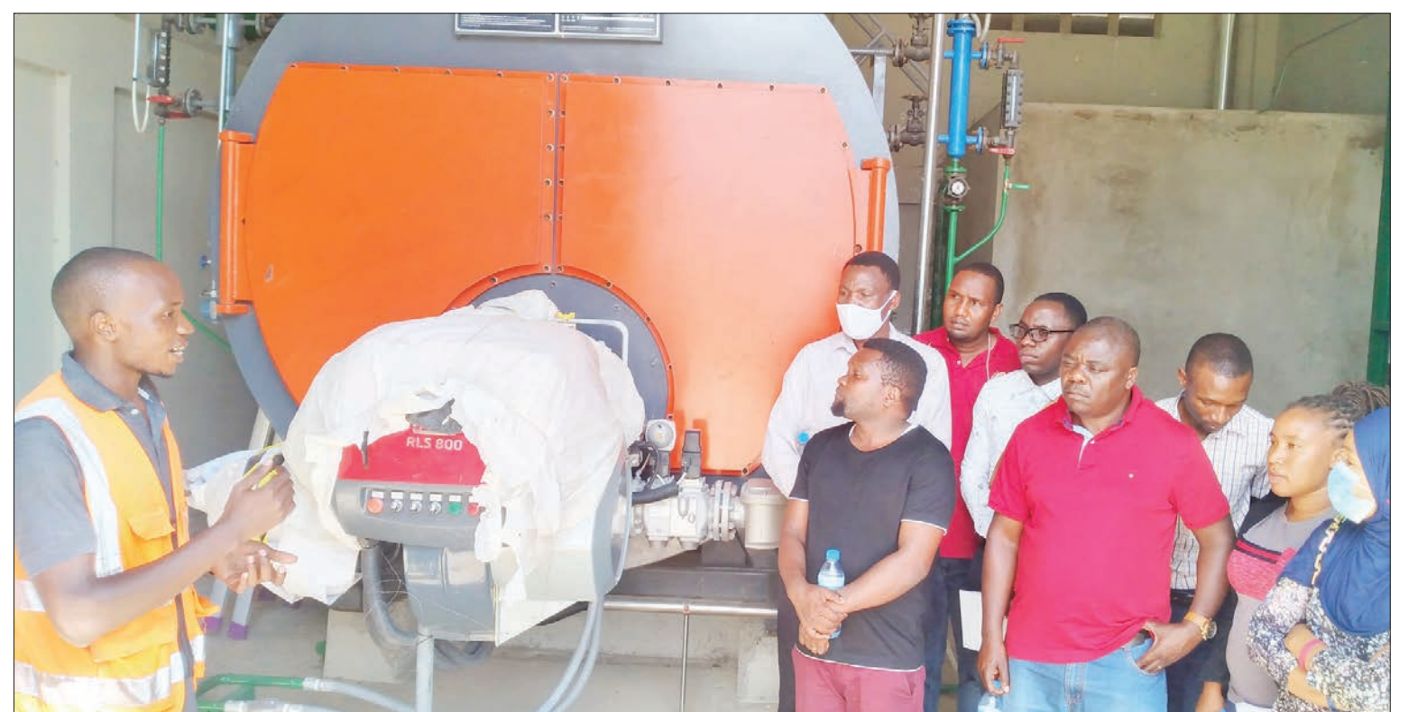
Peter Luhwago (L), a mechanical engineer with Kairuki Pharmaceuticals Industry Limited, briefs members of the Pharmaceuticals Society of Tanzania on a tour of the firm at Zegereni in Kibaha District at the weekend on one of the machines. Photo: Joseph Mwendapole
