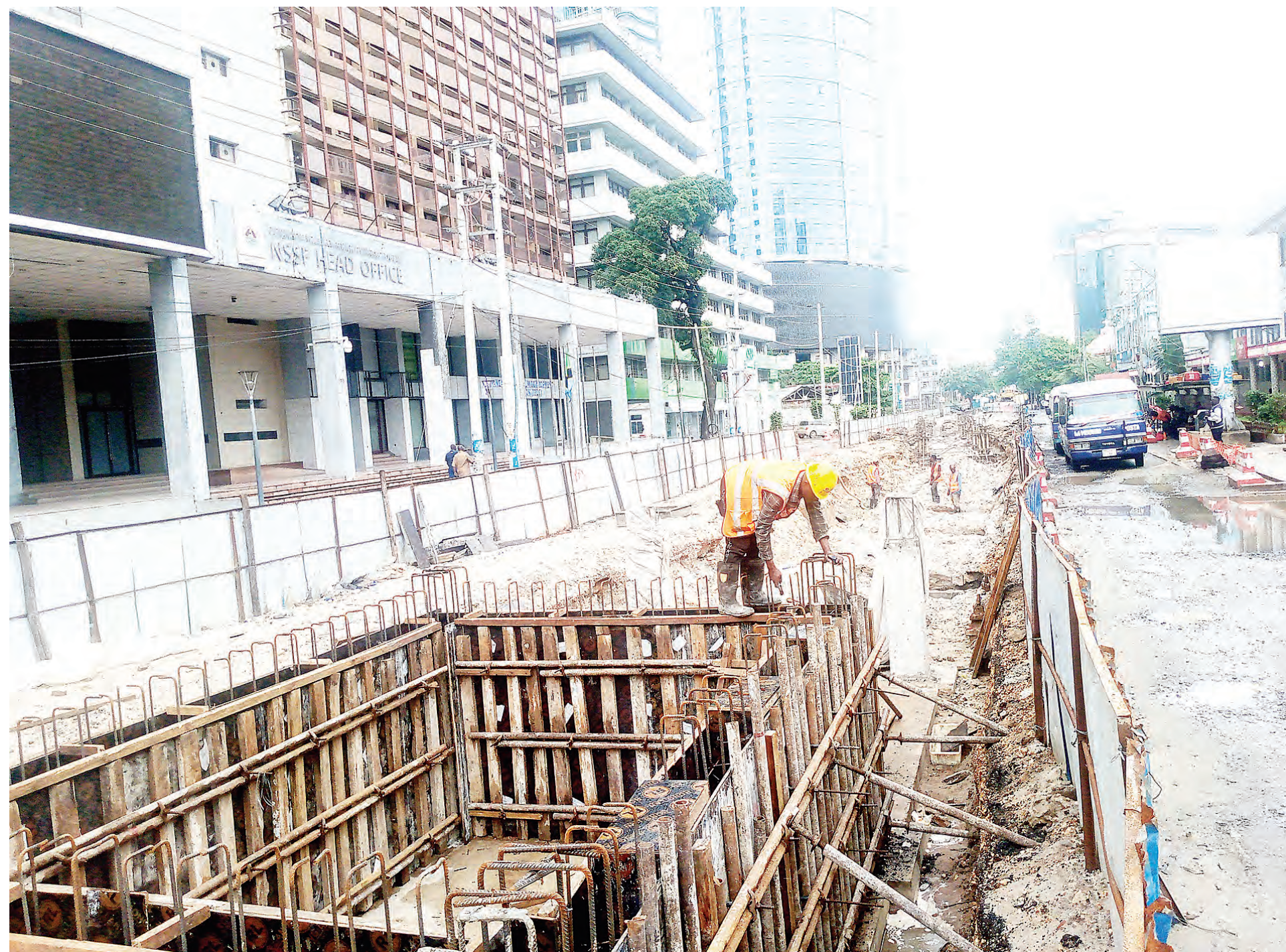
Construction of rapid transit bus station in progress near New Post Office in Dar es Salaam, as captured yesterday. Photo: Correspondent Sabato Kasika
