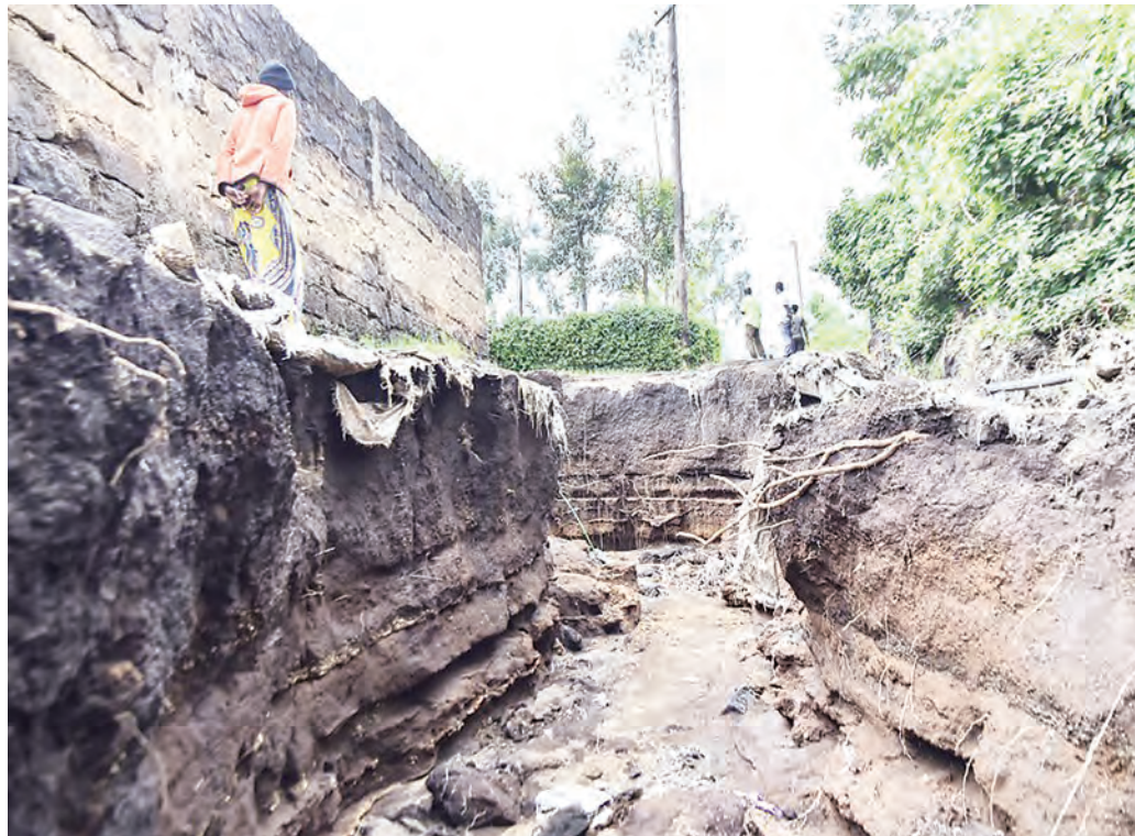
A woman walks beside a deep gully near a residential building in Rongai, Nakuru County, Kenya, May 7, 2024. Xinhua
