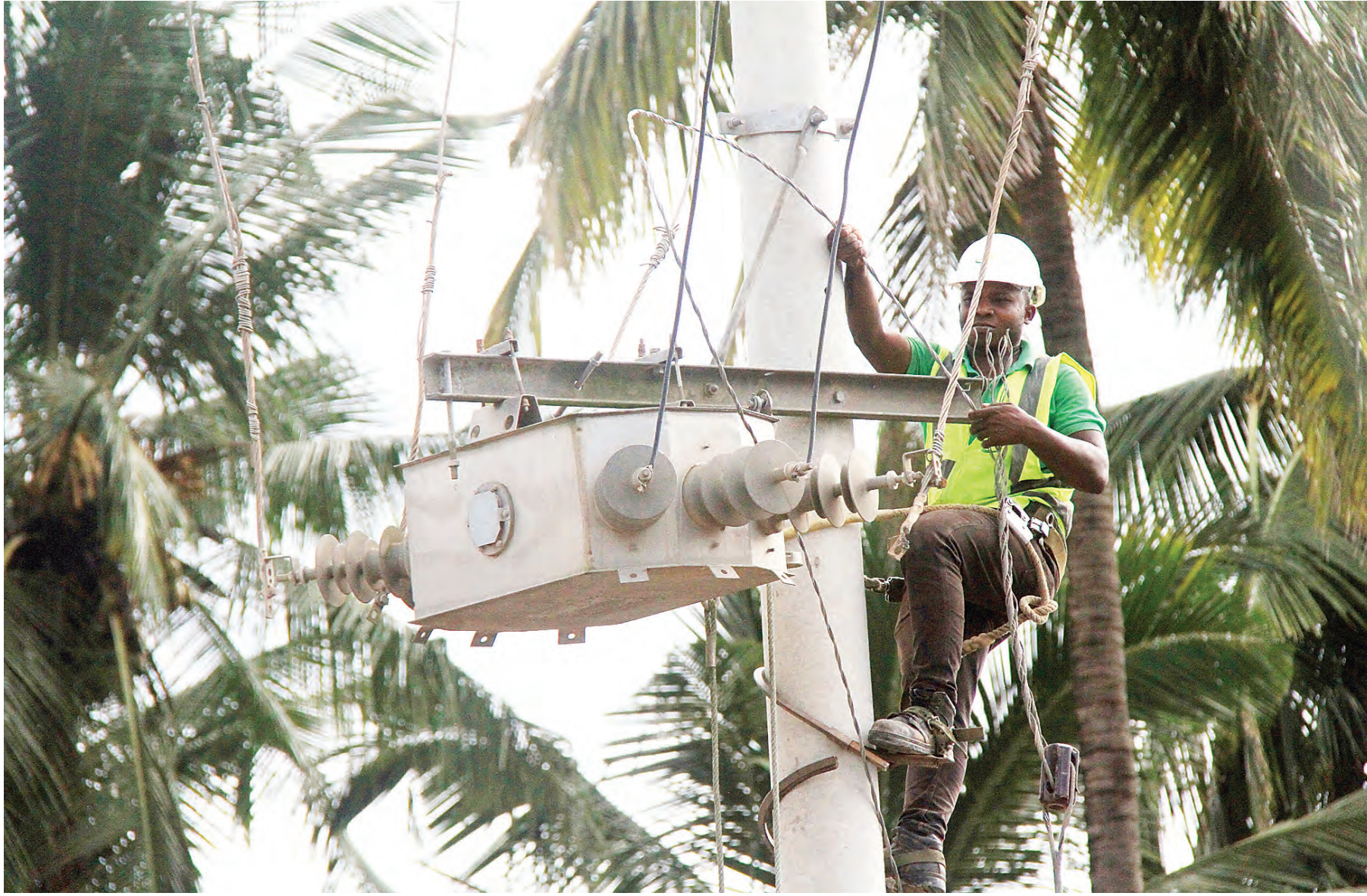
Tanzania Electric Supply Company Ltd (Tanesco) technician repairs high-tension power cables in Dar es Salaam's Kitunda suburb yesterday. Photo: Correspondent Jumanne Juma
