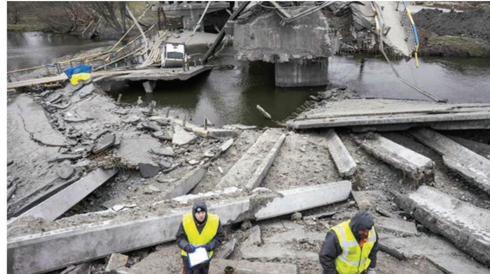
Engineers inspect the state of destruction of the bridge that connects Kyiv with Irpin, Ukraine, on Wednesday AP
