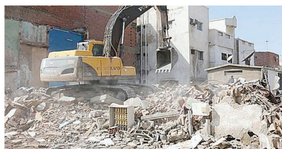
Demolition work is under way in Jeddah's 26 undeveloped districts as part of the city's major redevelopment.
