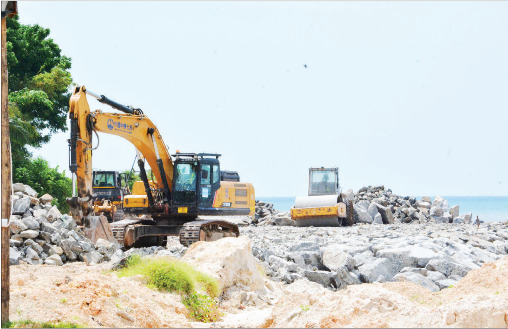
Land reclamation efforts well in progress yesterday along the Aga Khan Hospital stretch of Dar es Salaam's Indian Ocean coastline as the construction of a modern Selander Bridge to connect the area to Coco Beach continues. Photo: Correspondent Miraji Msala
