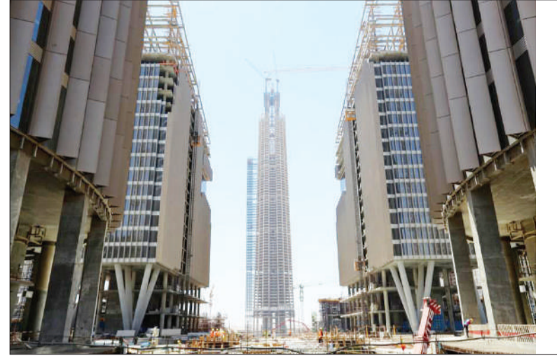
Photo taken on June 17, 2021 shows the construction site of a skyscraper in a vast business district in Egypt's new administrative capital. (Xinhua/Sui Xiankai)
