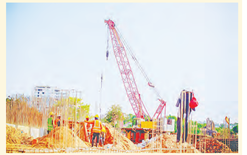
Ongoing renovations work on Kemondo Bay Port's depth and quay length. Photo: Guardian Correspondent
