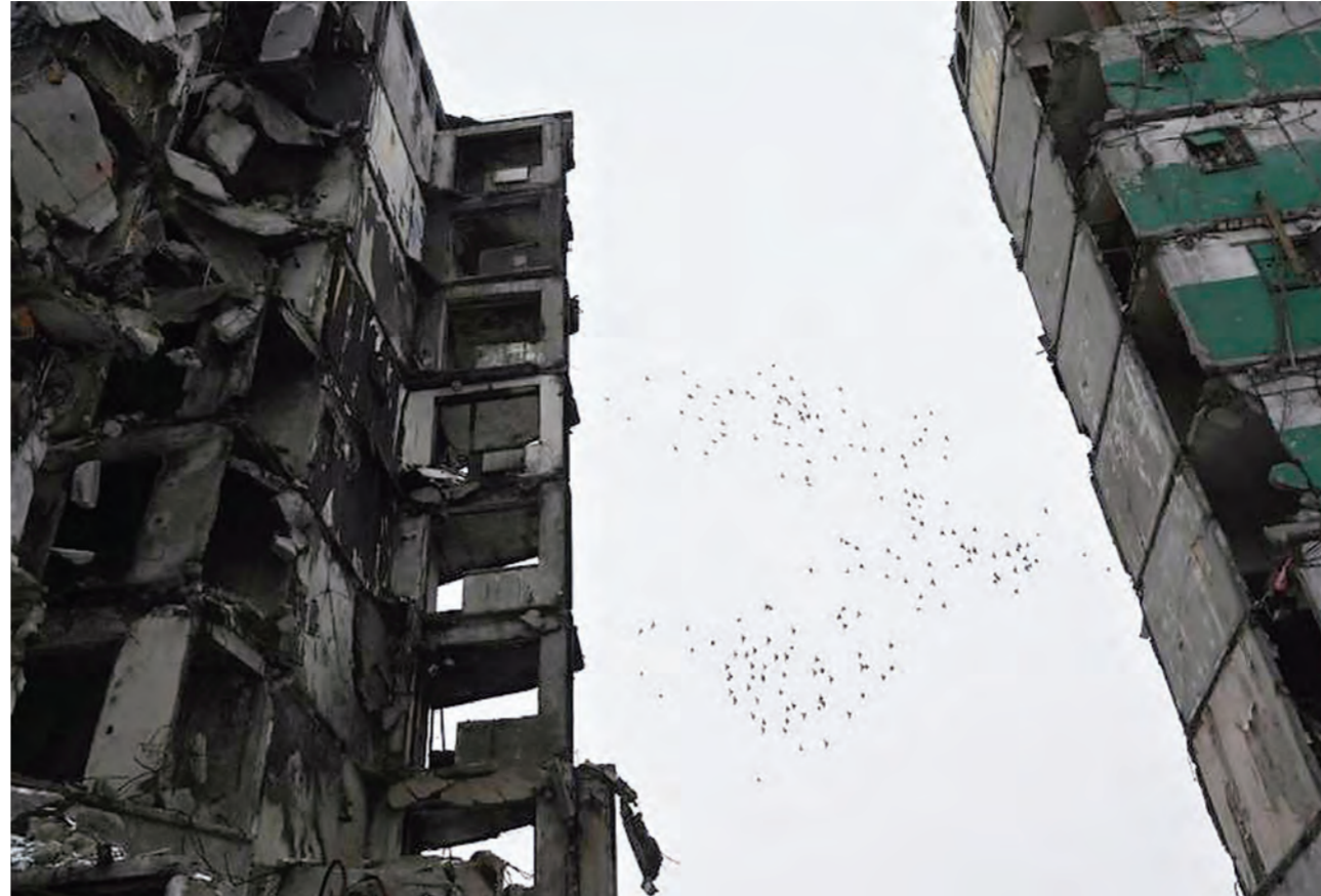
A flock of pigeons fly between two damaged buildings in the small Ukrainian town of Borodyanka, some 60 km from Ukrainian capital of Kiev on Jan 12, 2023. (PHOTO / AFP)
