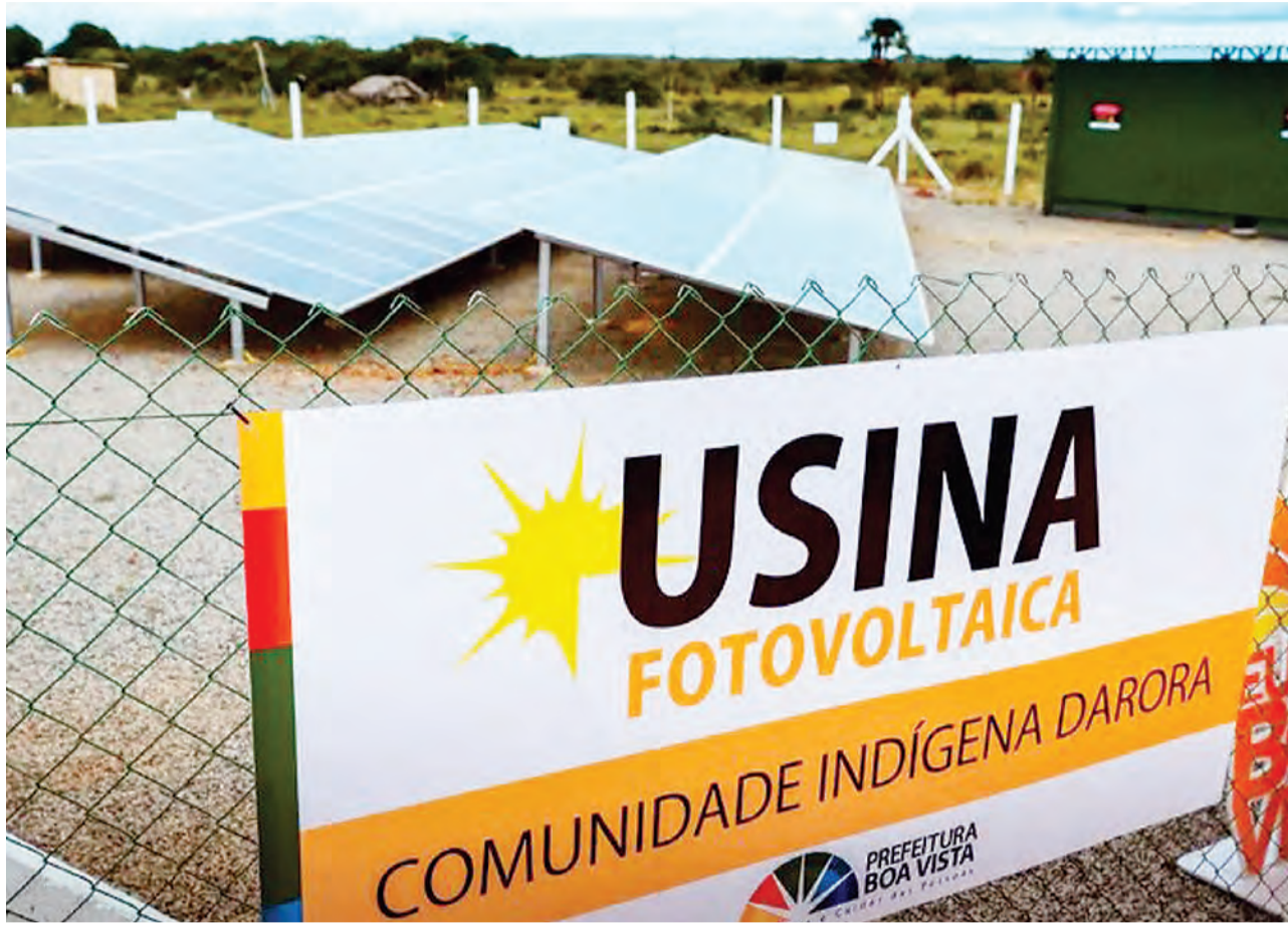
Solar panels with a capacity to generate 30 kilowatts no longer work in the Darora Community of the Macuxi people, an indigenous group from Roraima, a state in the far north of Brazil. The batteries only worked for a month before they were damaged because they could not withstand the charge. CREDIT: Boa Vista City Hall
