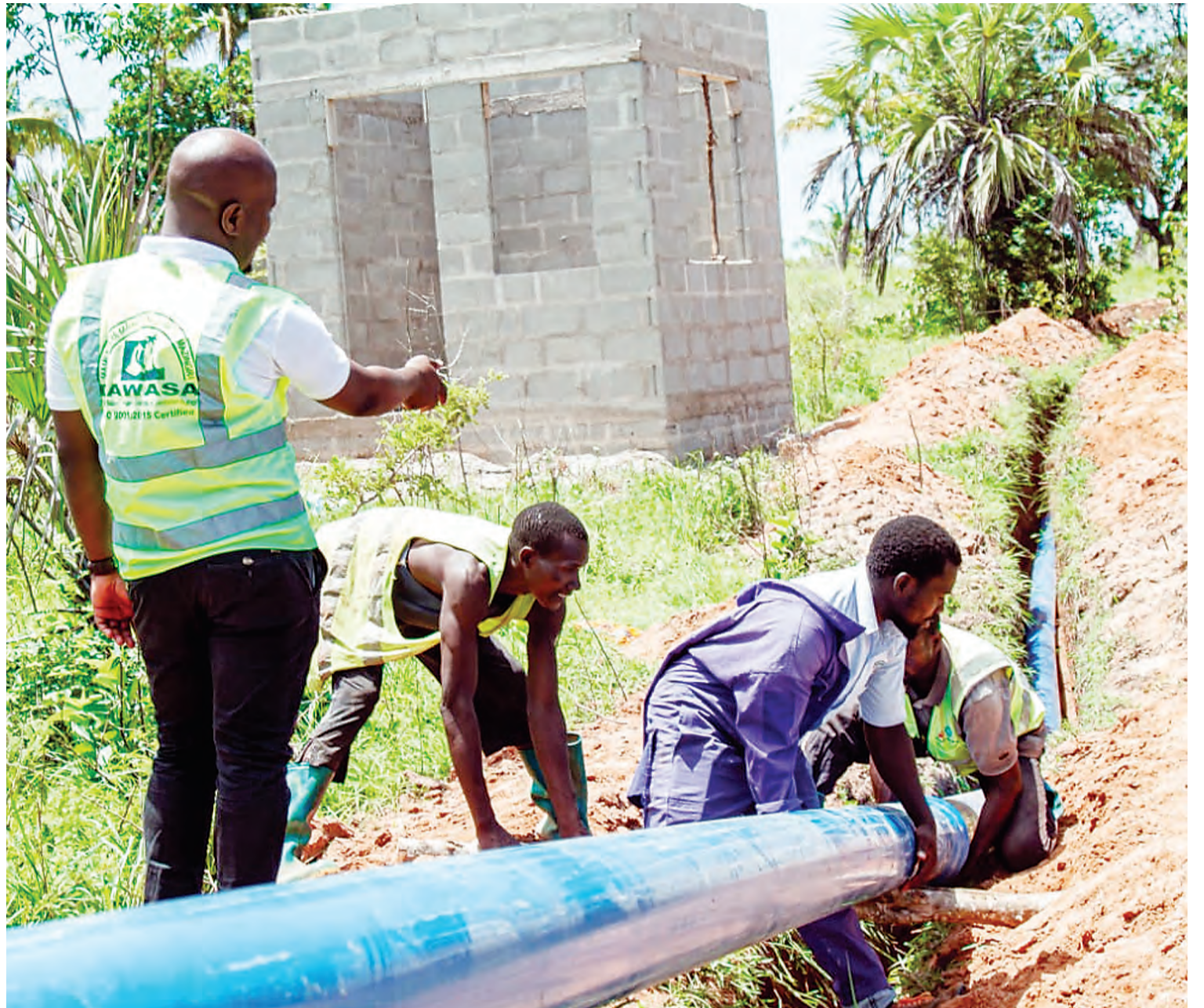
Dar es Salaam Water and Sanitation Authority (Dawasa) technicians lay a water pipe in Dar es Salaam's Mabwepande suburb on Thursday in implementation of the Mbopo Chekanao water project. Photo Correspondent Joseph Mwendapole
