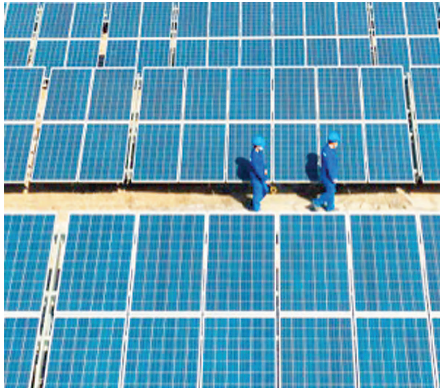
Technicians inspect and maintain photovoltaic panels in Yuli County, Bayingolin Mongol Autonomous Prefecture, northwest China's Xinjiang Uygur Autonomous Region, Feb. 25, 2021. File Photo
