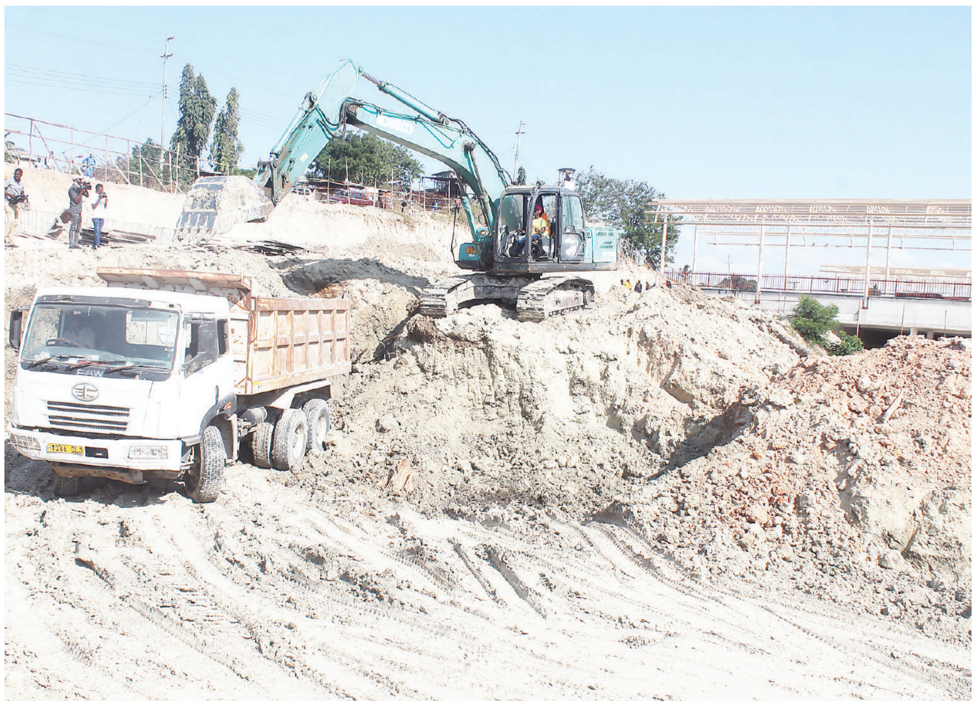
Construction of Dar es Salaam's Mbezi Mwisho upcountry bus terminal well under way, as found earlier this week. Photo: Correspondent Jumanne Juma
