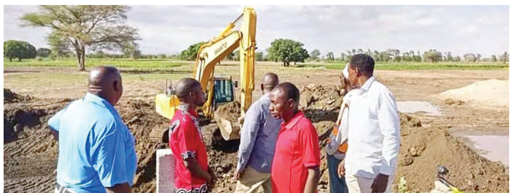
Village chairmen from Mirerani township in Simanjiro District on an inspection tour of Nduruma River dam and Kidawash canyon following recent floods in the area. Photo: Correspondent Gift Thadey
