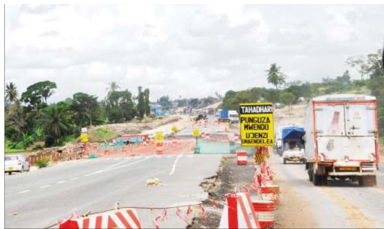
Motorists drive along a service road yesterday owing to the ongoing construction of a bridge at Mbezi Mwisho in Dar es Salaam being undertaken as part of the first phase of the expansion of the Kimara-Kibaha stretch of Morogoro Road into a six-lane carriageway. Photo: John Badi
