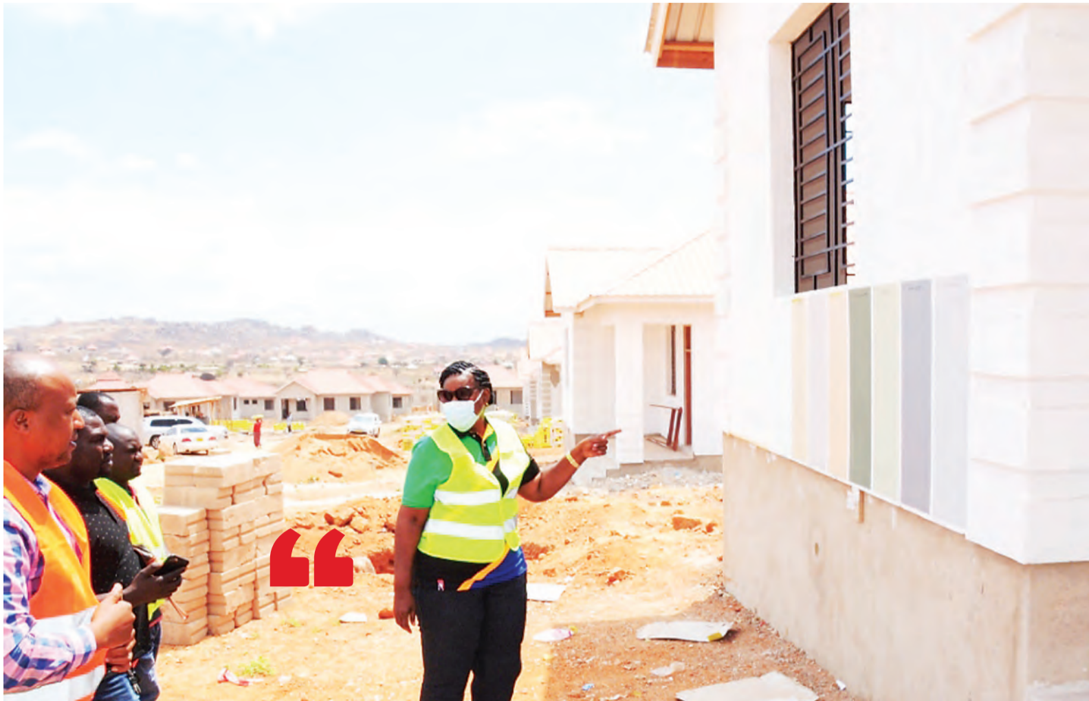
Dr Angelina Mabula, Deputy Minister for Lands, Housing and Human Settlements, pictured yesterday has a first-hand account of progress in the implementation of a project expected to see 300 houses built in Dodoma Urban District's Iyumbu administrative ward. Photo: Correspondent Munir Shemweta
