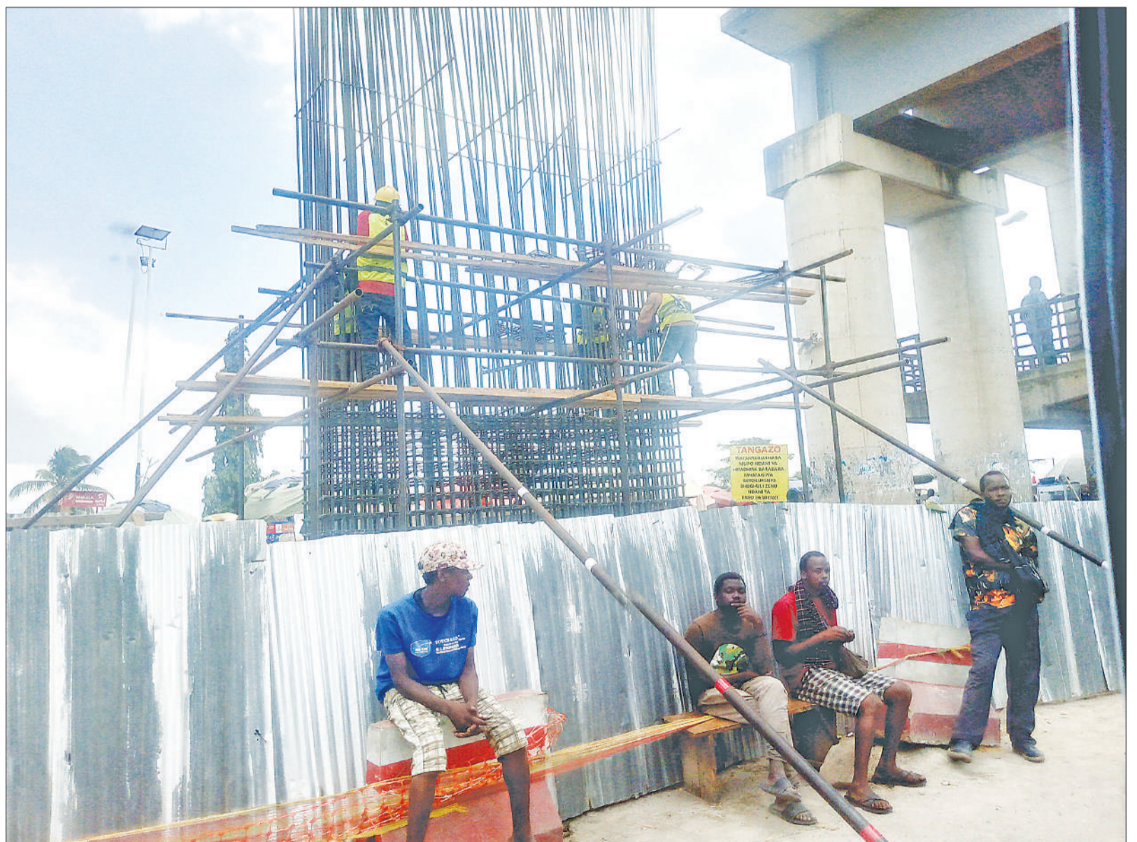
Construction of overhead bridge at a Kimara Mwisho suburb intersection of Dar es Salaam's Morogoro Road in progress, as found yesterday. Photo: Correspondent Sabato Kasika
