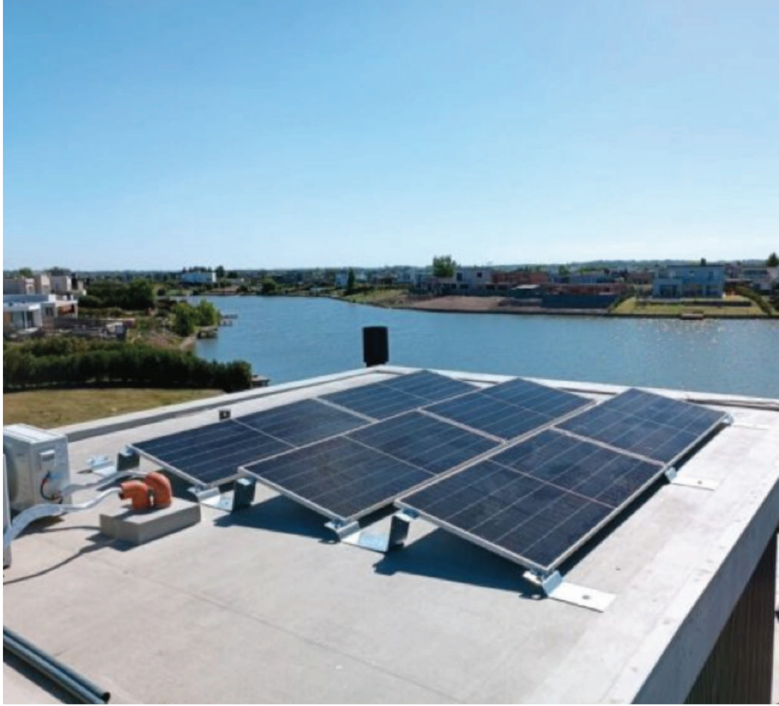
Aerial view of the 5000 square meter roof full of solar panels, in one of the pavilions of La Rural, the busiest fair and exhibition center in Buenos Aires. It is the largest private solar park in the capital of Argentina and required an investment of almost one million dollars.
