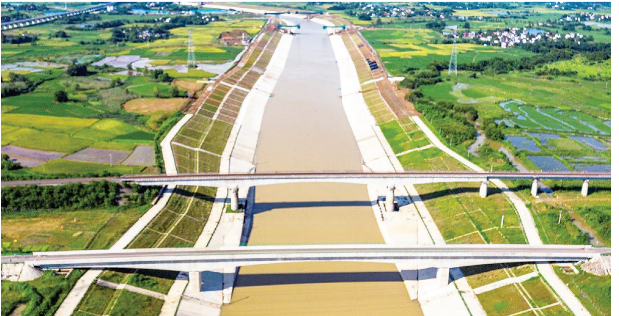
Photo taken in July 2021 shows a project diverting water from the Yangtze River to the Huaihe River in Ketan township, Lujiang county, Hefei, east China's Anhui province. File photo
