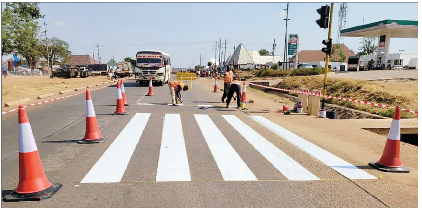
Tanzania National Roads Agency (Tanroads) employees busy working on a zebra crossing on a trunk road in Geita Region yesterday. They said it is an on-going activity. Photo: Correspondent Joctan Ngelyi
