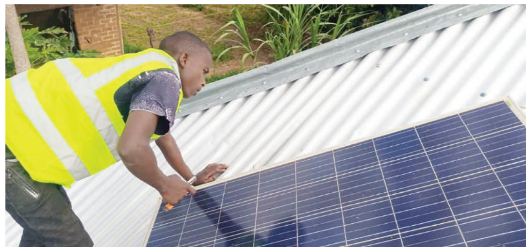
Kelvin Chengula on the rooftop of his client to install a solar panel PHOTO/A CORRESPONDENT
