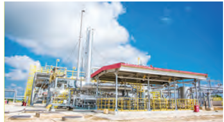
TPDC FOR CNG STATION, VEHICLE MODIFICATION WORKSHOP PAGE 4
