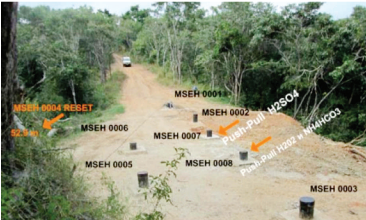
In-Situ Leaching test wells at Mkuju River uranium project in Tanzania. Source: Uranium One
