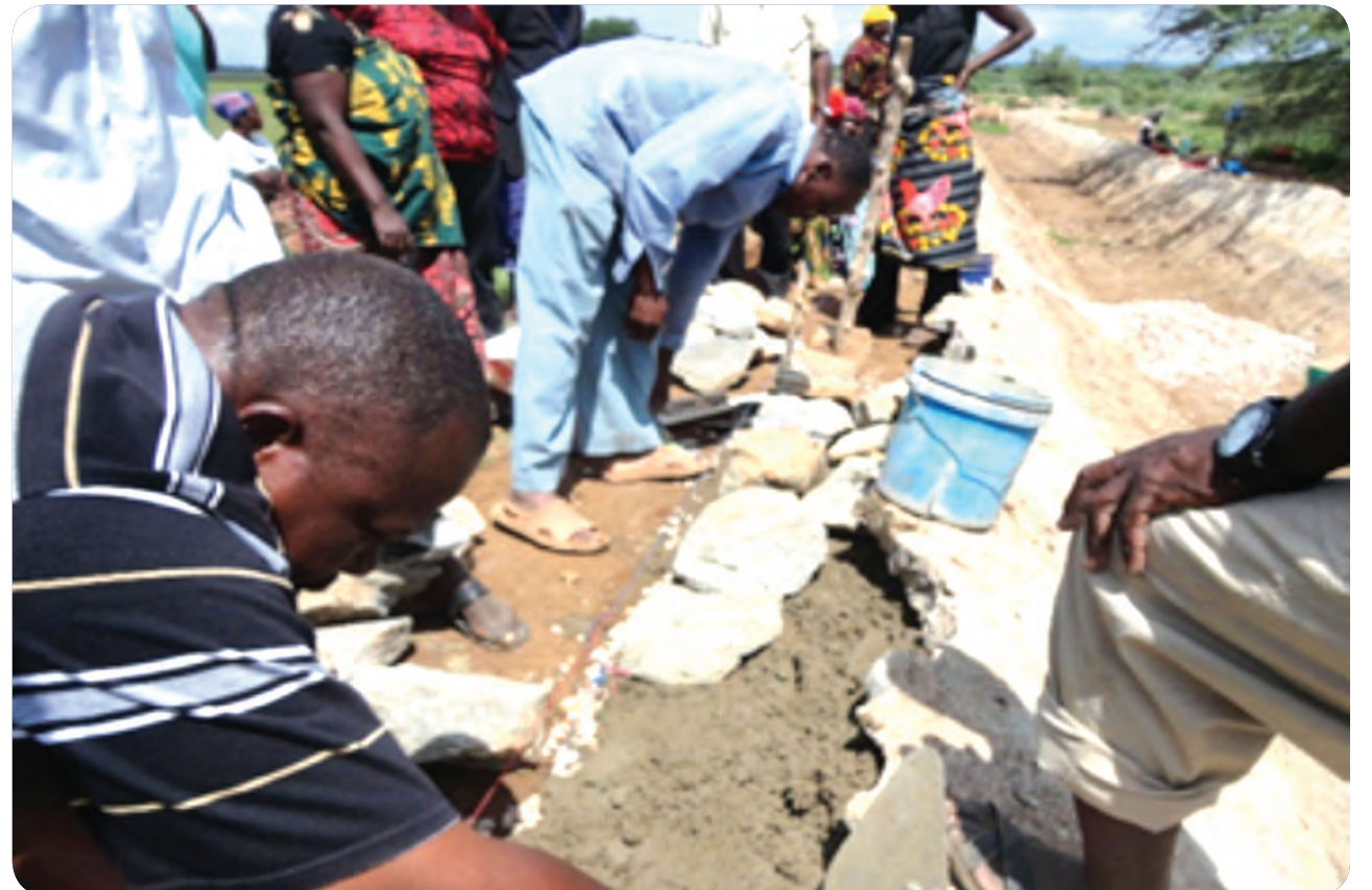
Participatory repair work of irrigation canal. 10 members implemented capping technically supported by district and zone staff.
