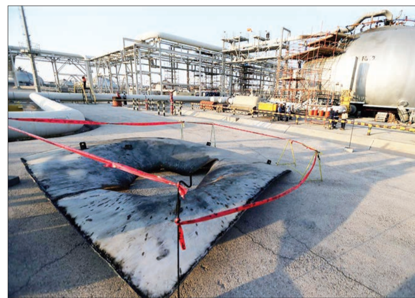
A metal part of a damaged tank is seen at the damaged site of Saudi Aramco oil facility in Abqaiq, Saudi Arabia, on Saturday. REUTERS
