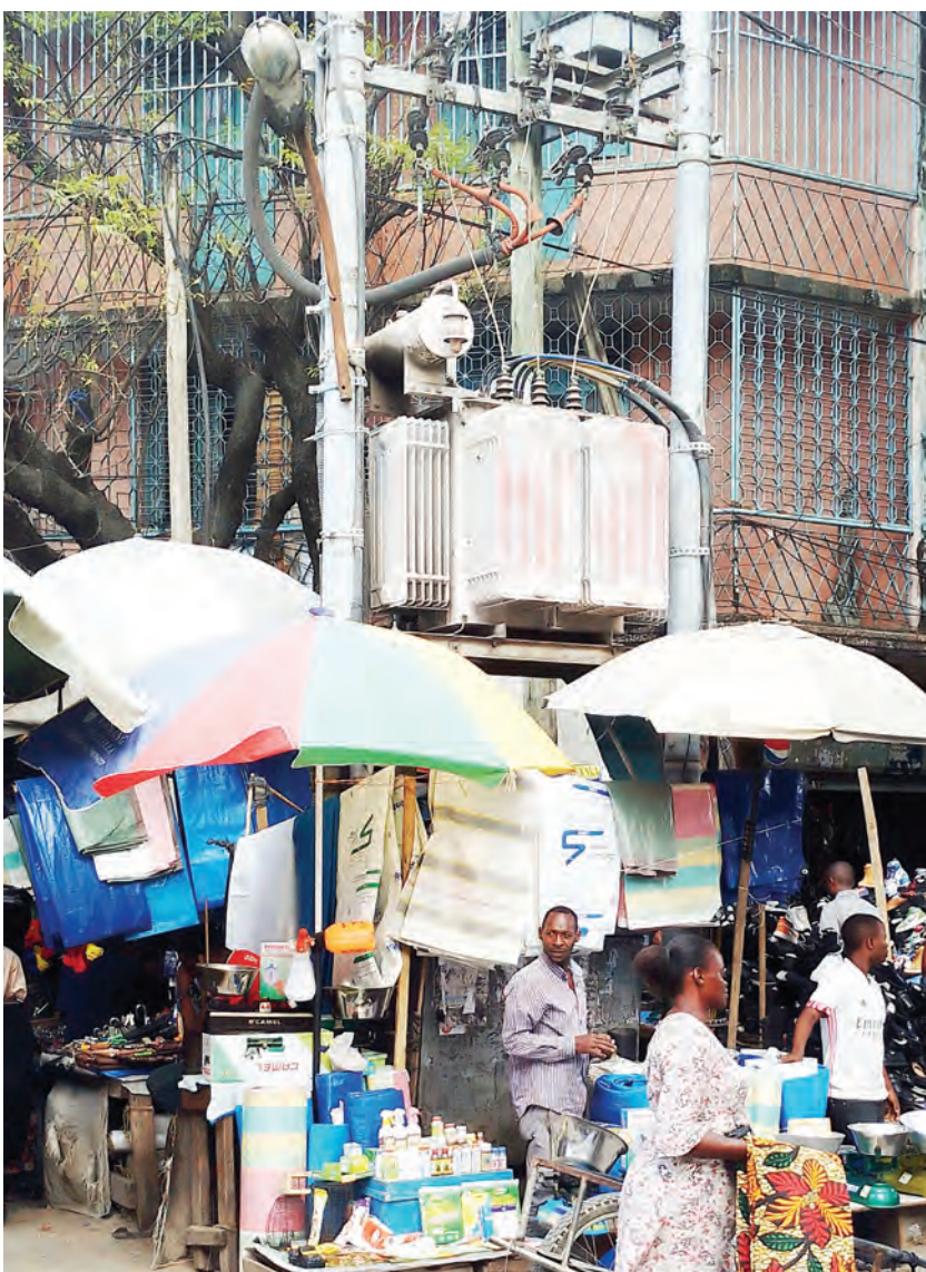
Small traders at high risk as they conduct their activities just next to a high-voltage transformer at the Tandamti Street/Nyamwezi Street intersection in Dar es Salaam's sprawling Kariakoo market zone yesterday. Despite the obvious danger, the scenario is far from rare in some urban areas in Tanzania. Photo: John Badi
