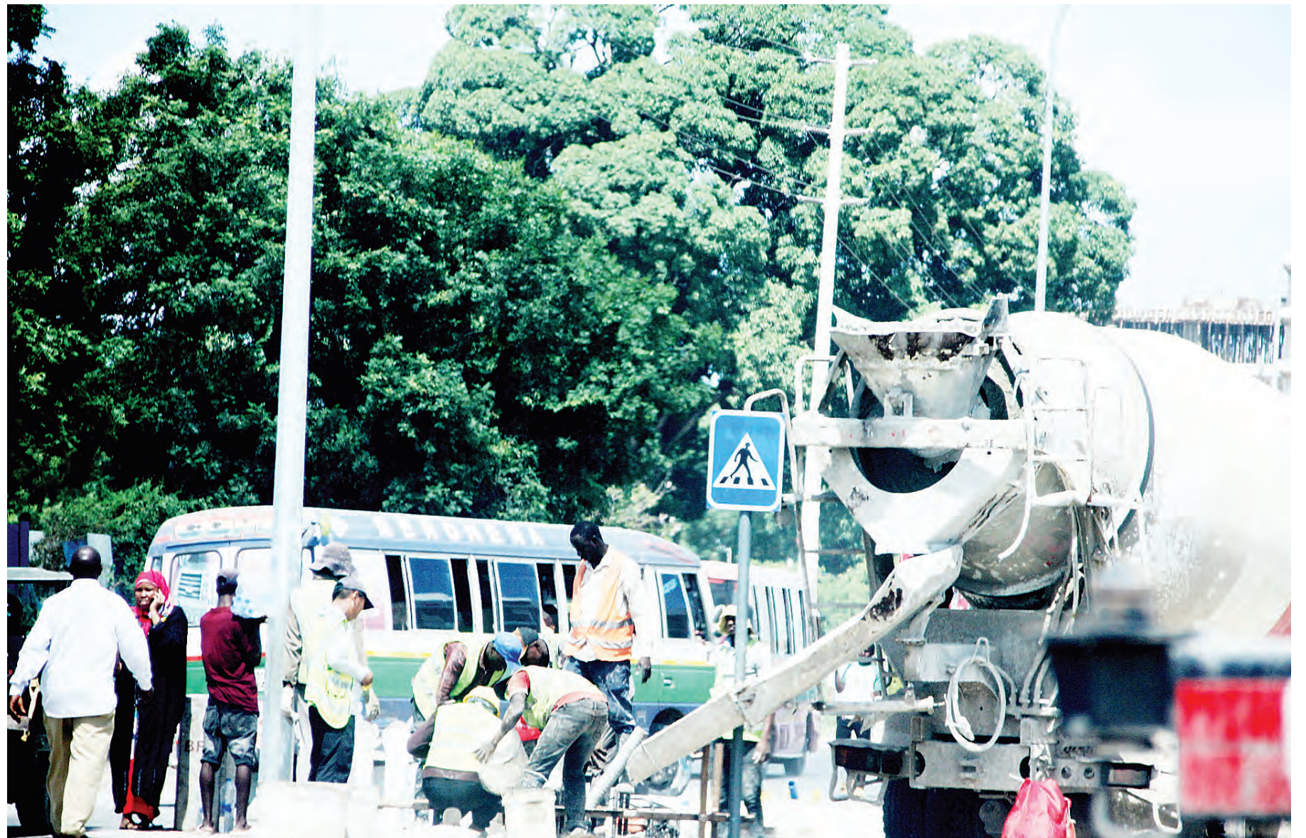
Work on a drainage chamber in progress yesterday at a Mbagala section of Dar es Salaam's Kilwa Road as part of the ongoing implementation of the city's rapid transit bus project. Photo: Correspondent Jumanne Juma
