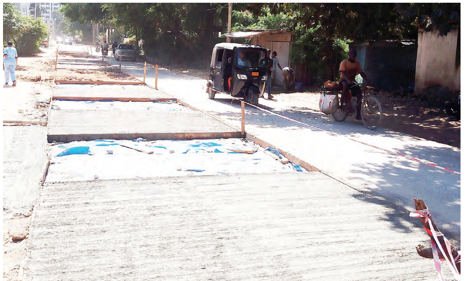
A section of Kalenga Street Road in Dar es Salaam's Upanga West suburb undergoes rehabilitation in the wake of massive damage mainly due to the recent heavy rains. Photo: John Badi
