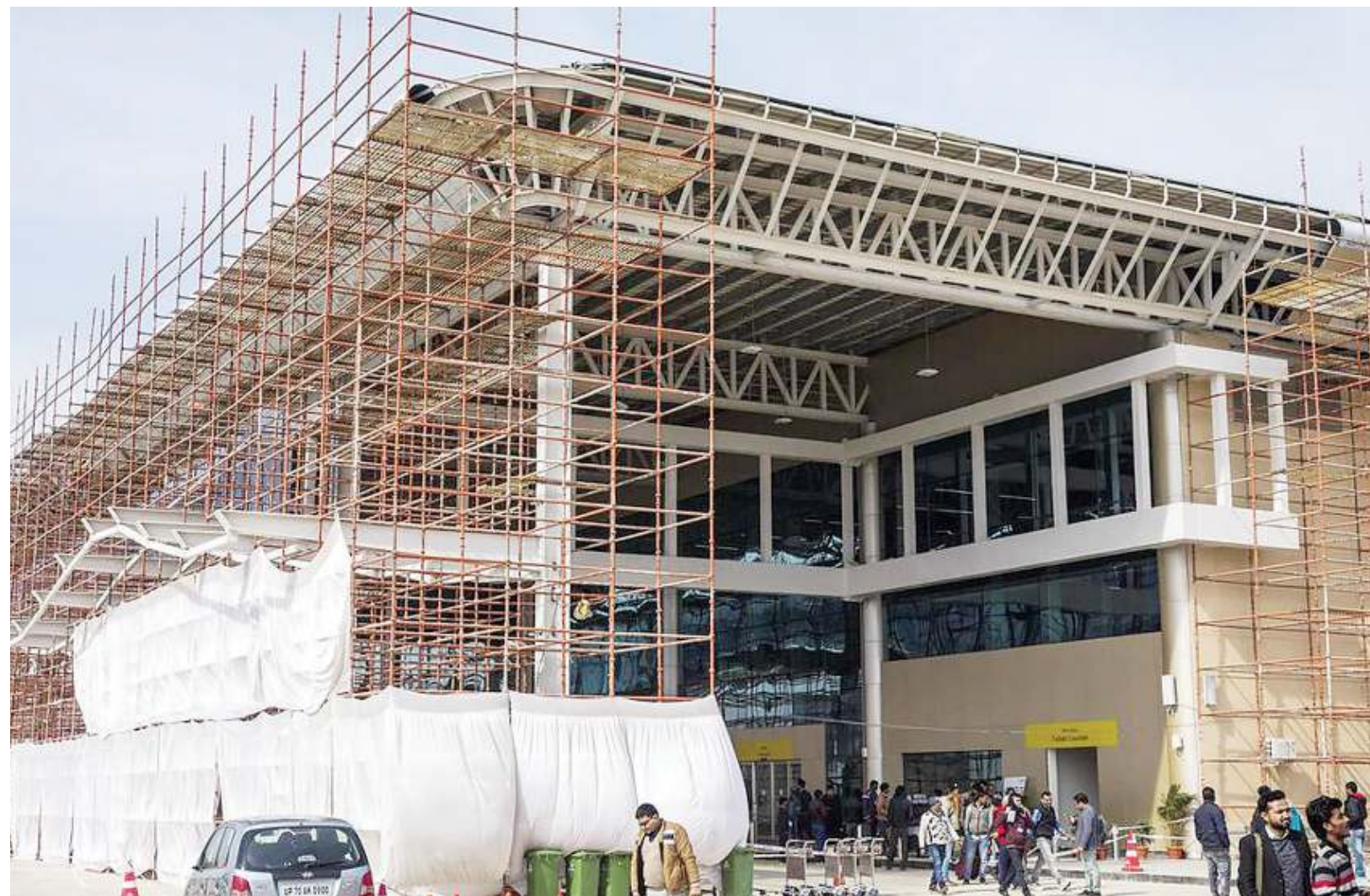
New building in Uttar Pradesh, India. The country's developers could be left facing tough times.
