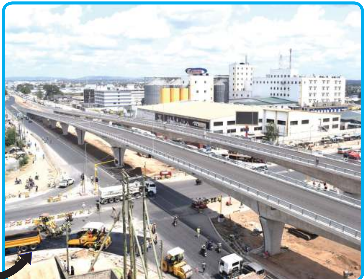
The overview of the constructed Mfugale flyover. Now 4 lanes are open for public use.
