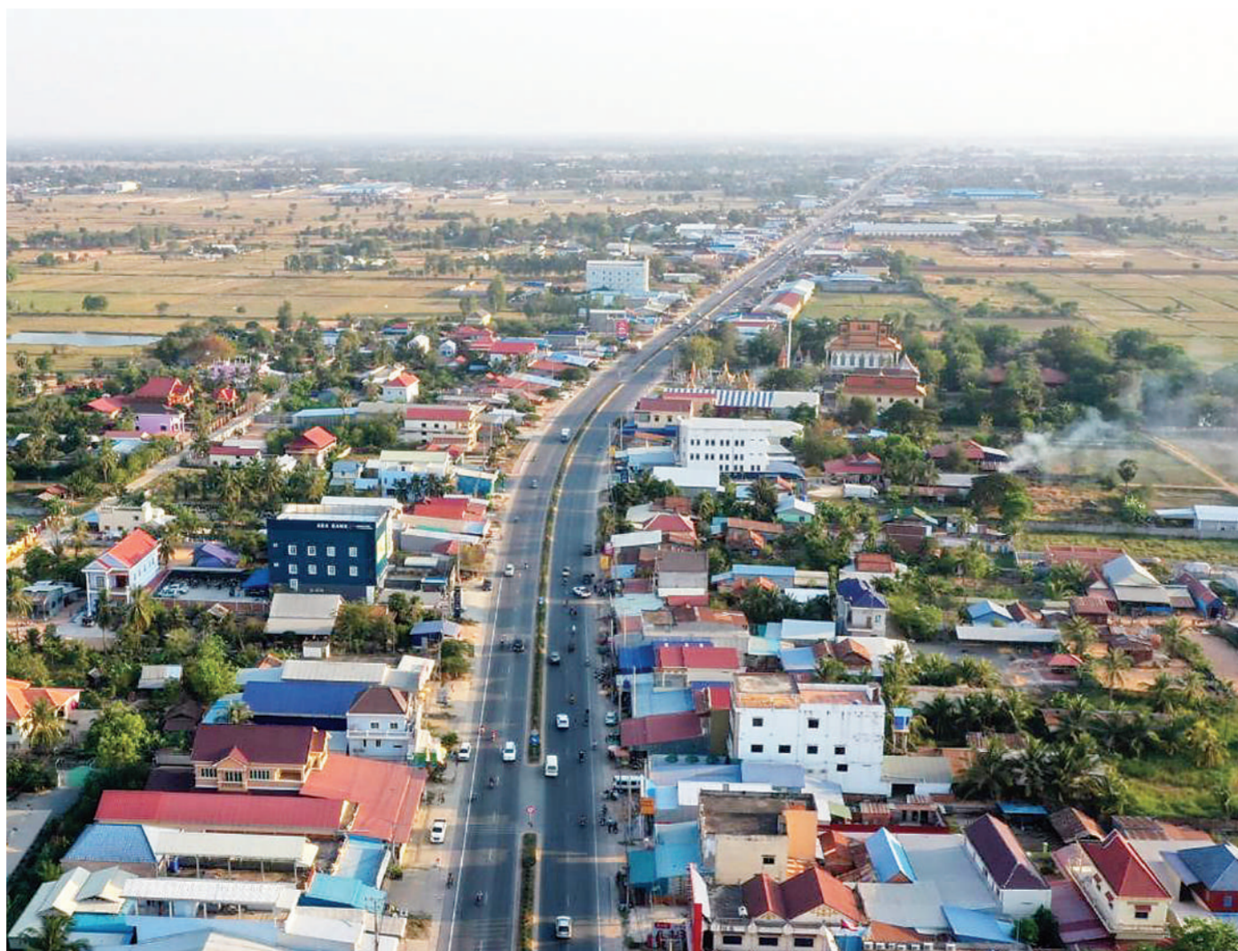
Photo taken on March 1, 2022 shows an aerial view of the China-funded National Road No. 3 reconstruction and expansion project in Takeo province, southern Cambodia. (Photo/Li Lai)
