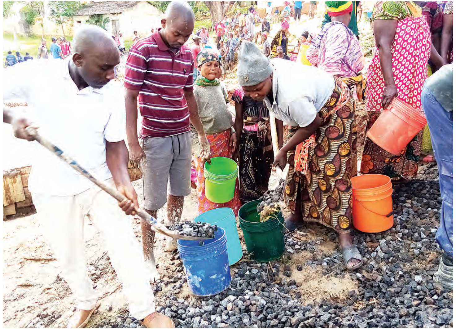
Japhet Hayule (L), a division officer in Muheza District, takes part in the building of classrooms and a teachers' office for Magila Secondary School earlier this week. Photo: Correspondent Steven William
