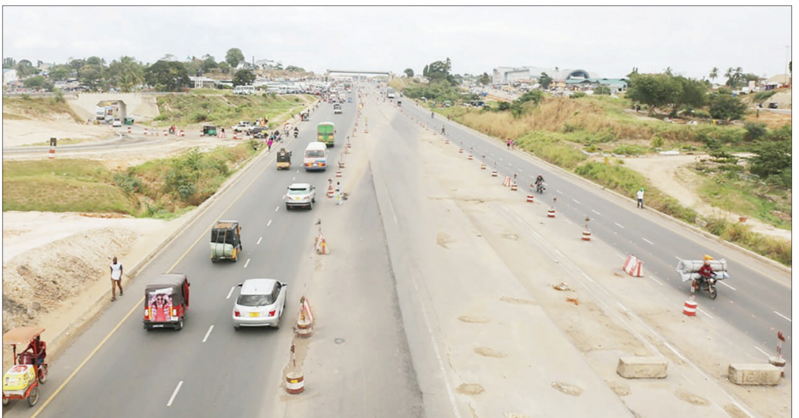
An aerial view captured yesterday of a section of the eight-lane 19.2-km highway between Dar es Salaam's Kimara suburb and Kibaha in Coast Region, with construction yet to be completed. Photo: Correspondent Shukuru Senkondo
