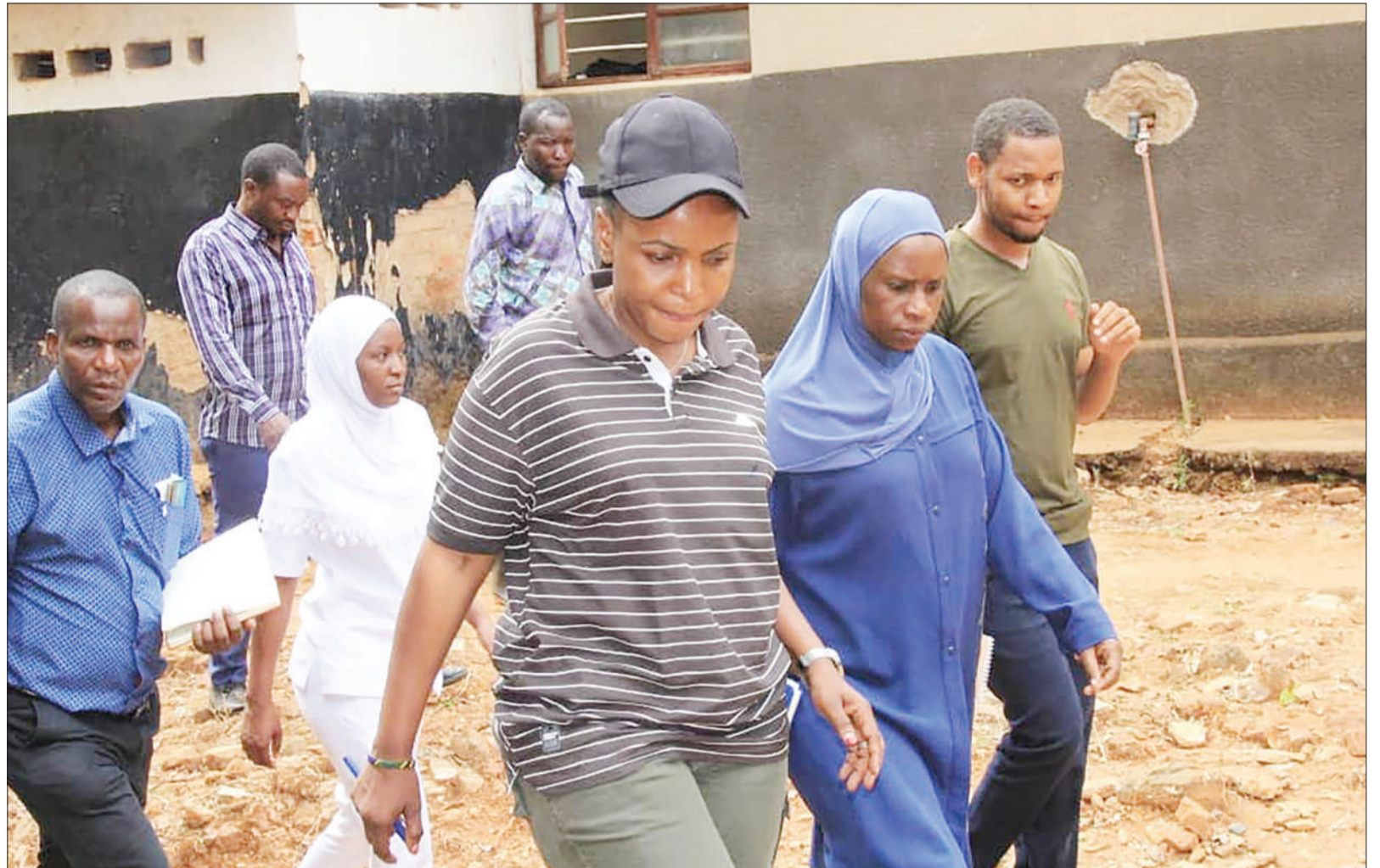
Songwe Region Administrative Secretary, Happiness Seneda (in a cap) inspects the construction of dispensary in Ileje District yesterday. She was unhappy that some equipment had been stolen from the construction site. Photo: Correspondent Ibrahim Yasin
