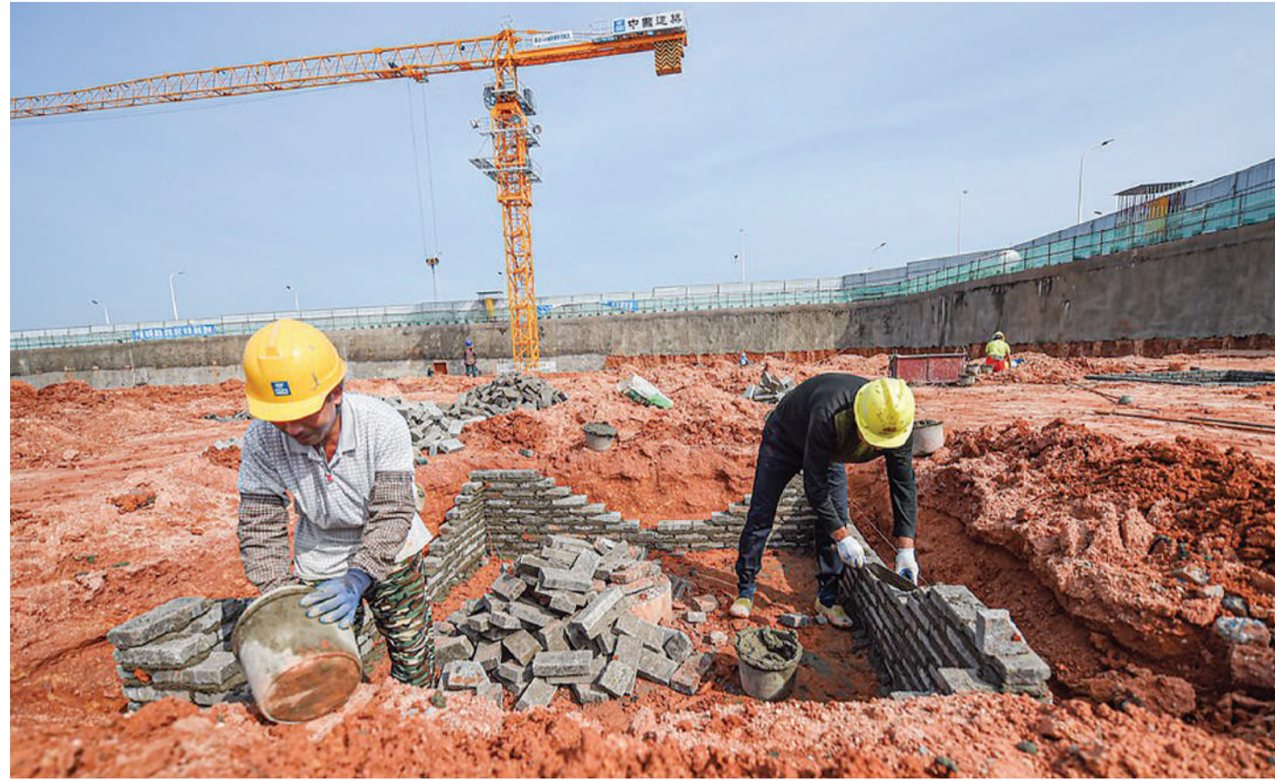
People work at the construction site of the West-coast Internet Headquarters Base in Haikou, south China's Hainan Province, Oct. 21, 2020. (Xinhua)
