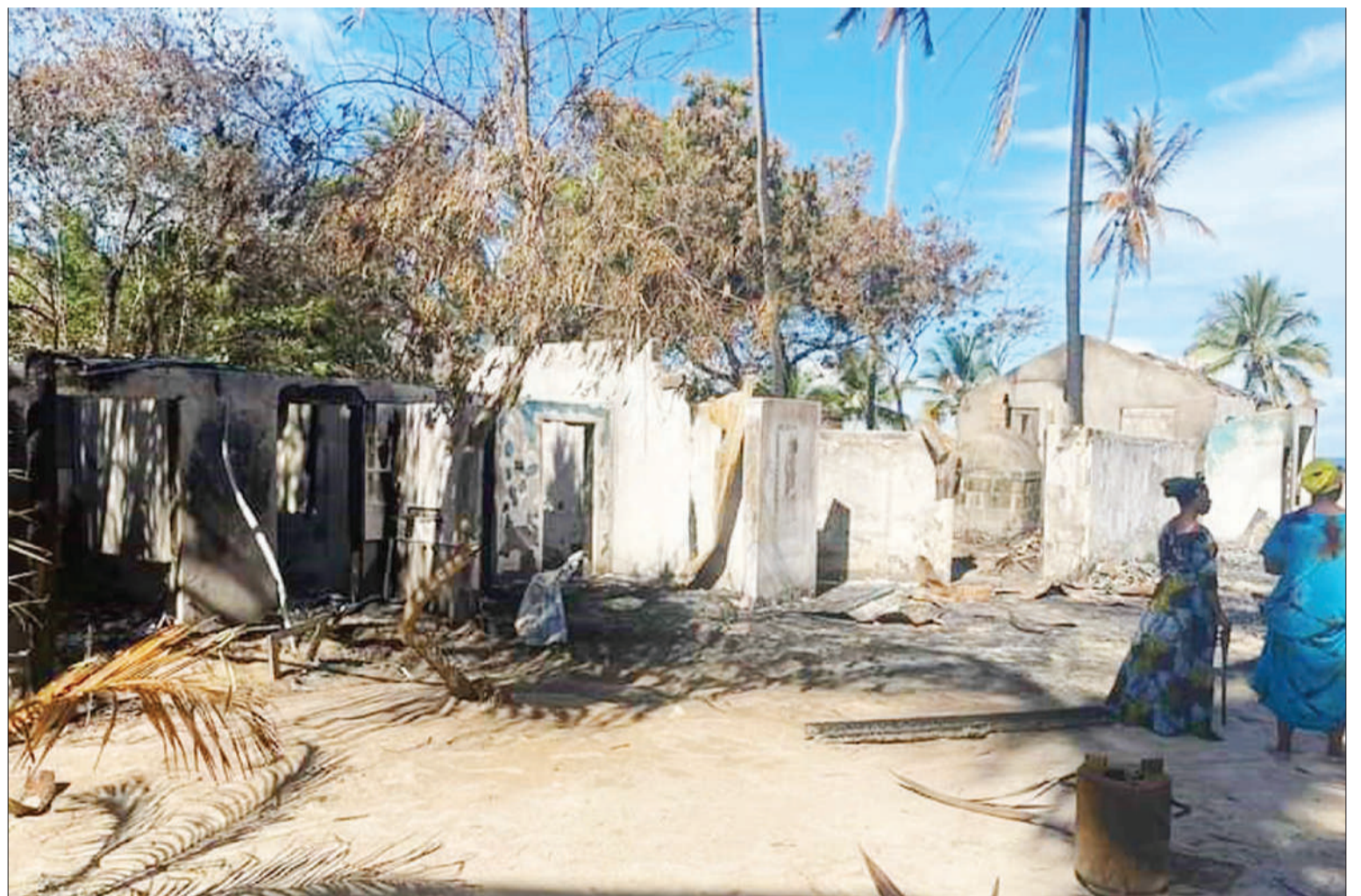
The remains of Mike's beach hotel cottages after having been destroyed by fire at Ushongo Beach village in Pangani District, Tanga Region over the weekend. Photo: Correspondent Steven William
