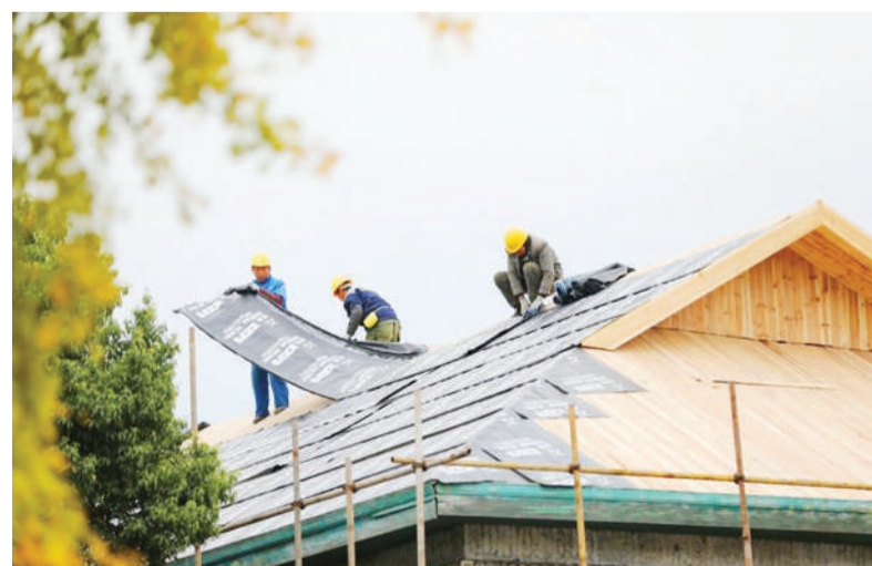
Photo taken on Dec. 4, 2020, shows workers renovating the roof of an old house in a residential complex in Daoxian county, Yongzhou, central China's Hunan province. Daoxian county promoted the renovation of old urban residential areas in 2020. (Photo by He Hongfu/People's Daily Online)
