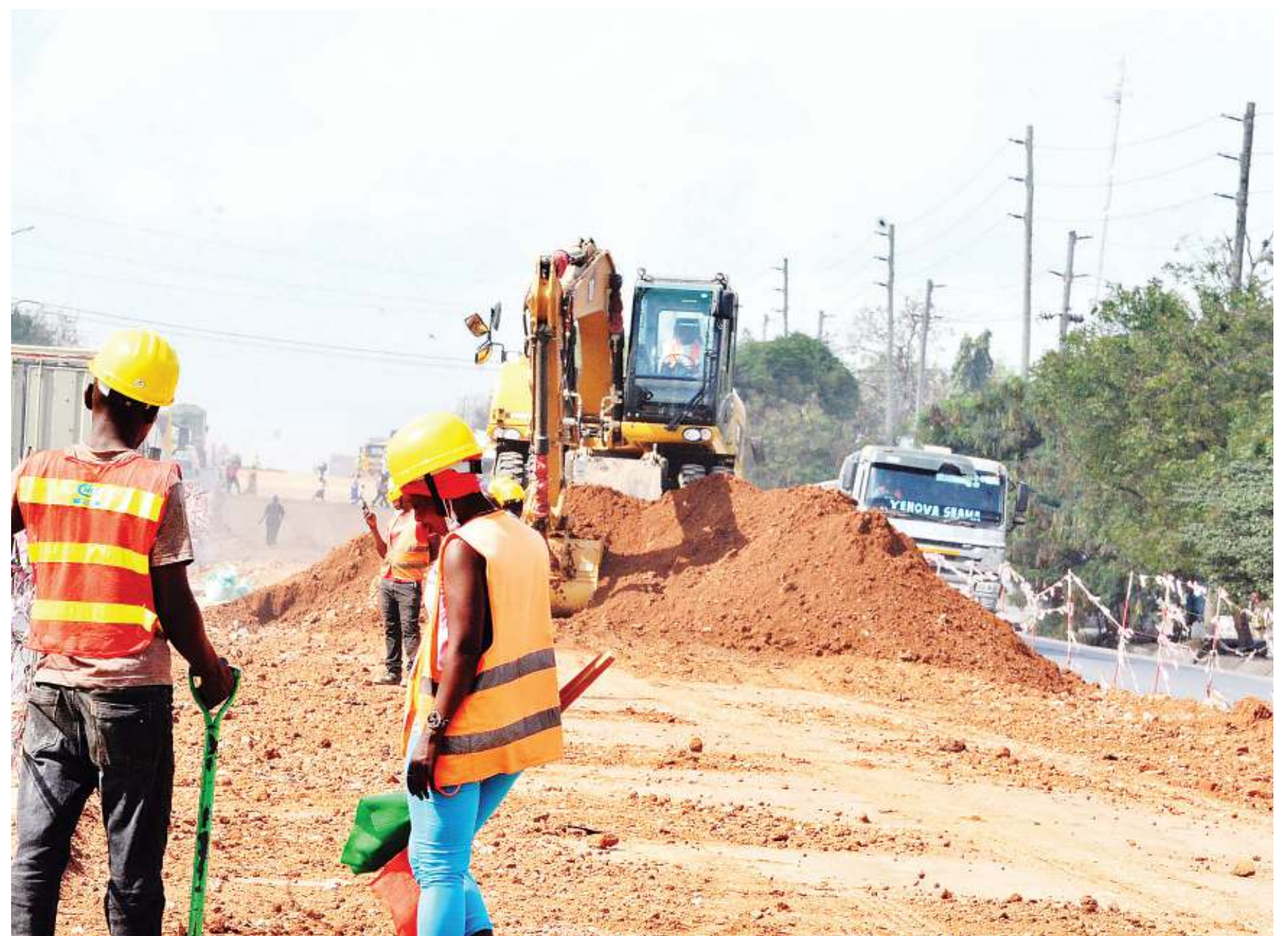
Implementation of the Dar es Salaam rapid transit bus infrastructural project has begun in earnest along the city's Kilwa Road, as found at Mabagala Kizuiani yesterday. Photo: Correspondent Miraji Msala
