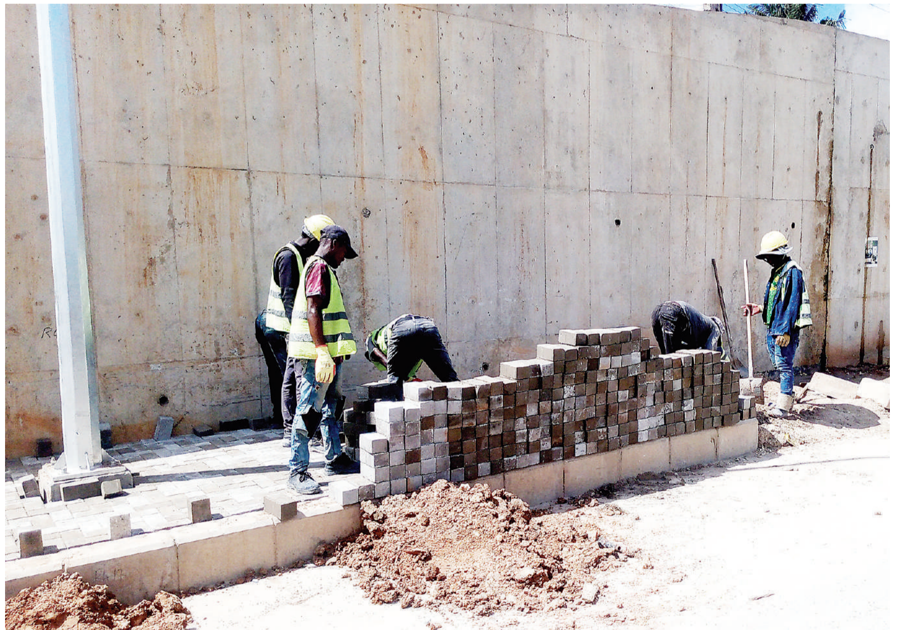
Improvement of roadside infrastructure on Dar es Salaam's ongoing Bus Rapid Transit project in progress yesterday along the Msimbazi stretch. Photo: Correspondent Sabato Kasika
