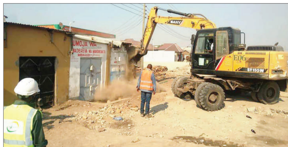
Tanzania National Roads Agency (Tanroads) officers in Mbeya Region pictured on Wednesday demolishing houses in Mbalizi in Mbeya Urban District said to be standing in road reserve reportedly while their owners have reportedly already been paid compensation and ought to have relocated. Photo: Correspondent Nebart Msokwa
