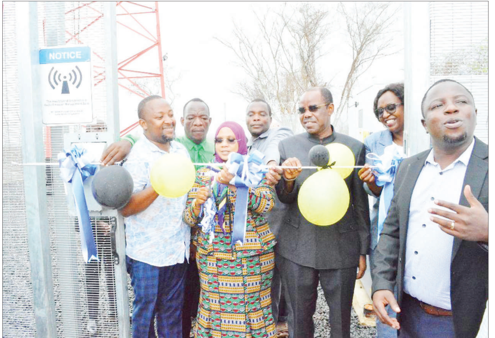
Dr Ashatu Kijaji, Minister for Information, Communications and Information Technology, cuts ribbon to launch the installation of a 4G telecommunication tower at Matuli village in Morogoro Region yesterday. The tower, mounted jointly by Airtel Tanzania and Universal Communication Services Access Fund, is meant to serve over 9,000 residents of Matuli, Kwaba, Diguli and Lulongwe villages. Photo: Guardian Correspondent
