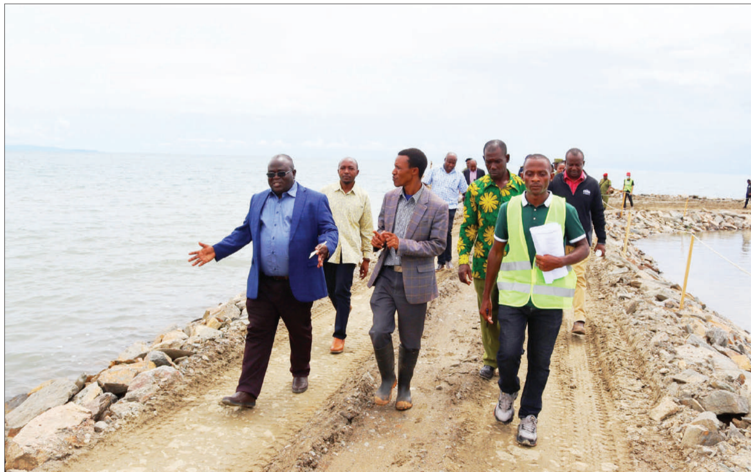
Works and transportation deputy minister Godfrey Kasekenya (L) has a word with Tanganyika district commissioner Salehe Mhando (C, foreground) after visiting Kalemii port construction site in Katavi Region at the weekend. Photo: Guardian Correspondent
