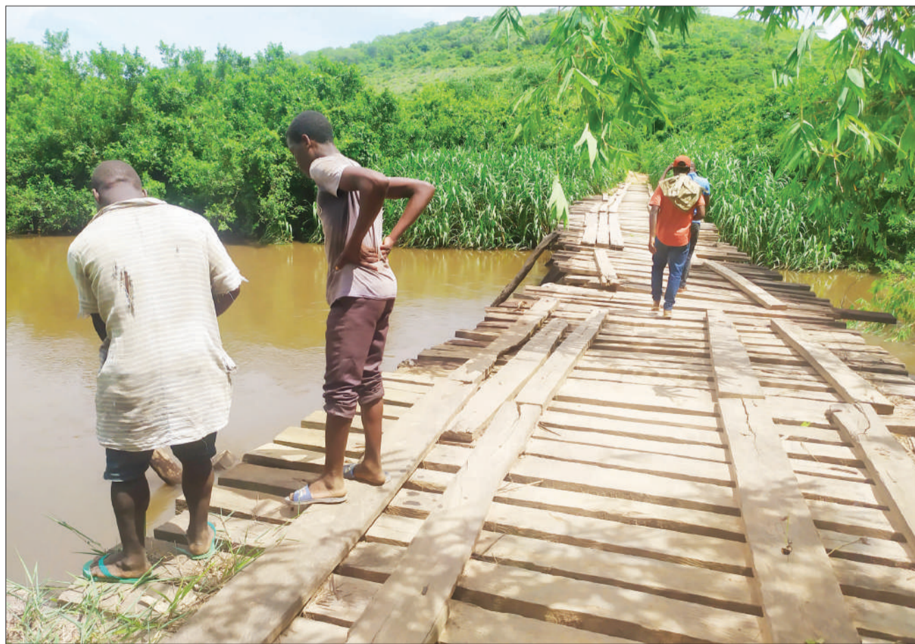
The Tanzania Rural and Urban Agency is reported to be lining itself up to build a permanent bridge to replace this one - across Mfuji River a strategic link for Tanganyika, Masagati and Mfenesi villages in Morogoro Region. Photo: Correspondent Idda Mushi
