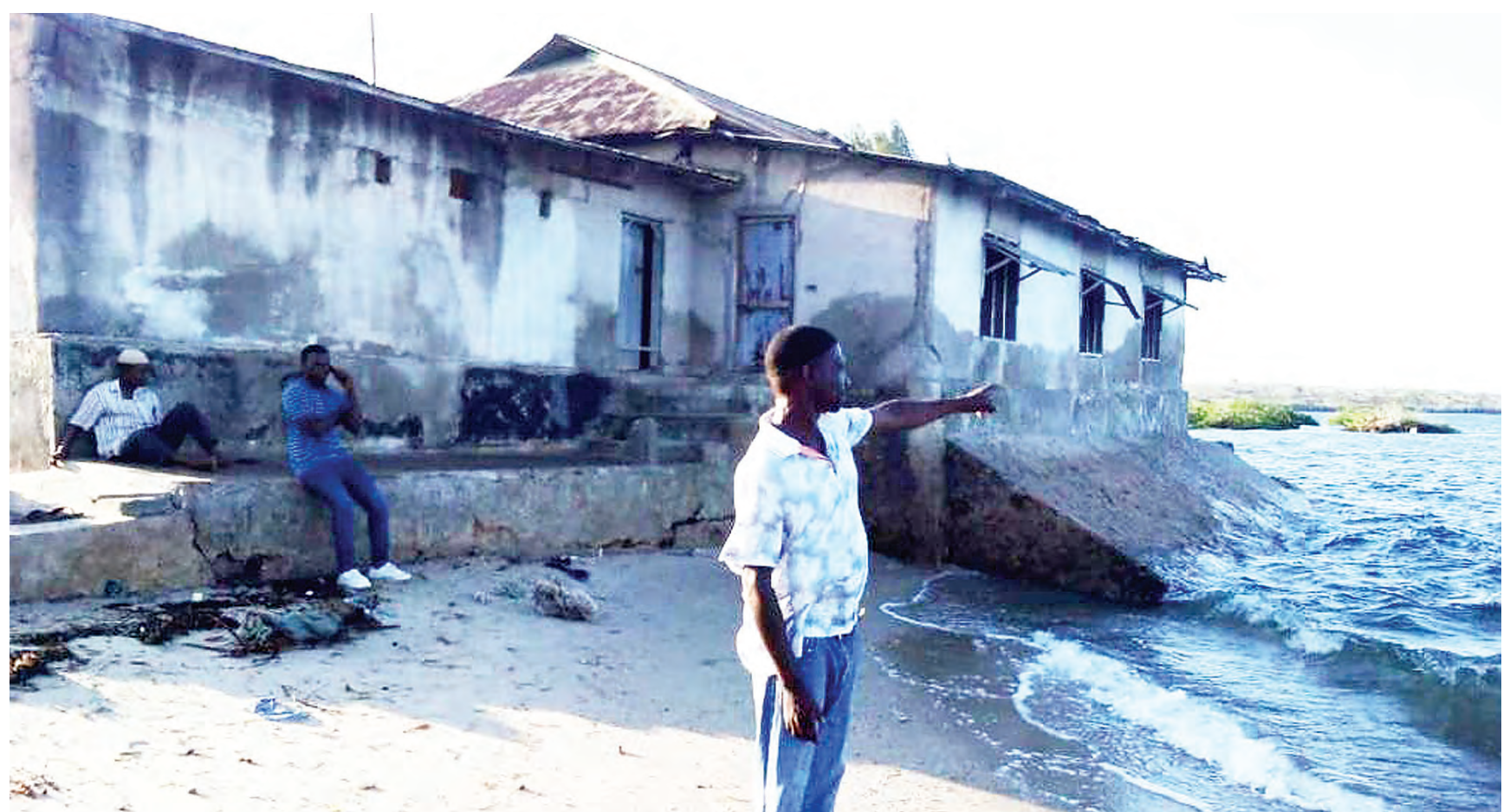
Msham Abdallah of Kisungure A at Mikindani Mtwara Region shows how seawater destroyed the Rehman Mosque building as a result of environmental degradation. Photo: Guardian Correspondent
