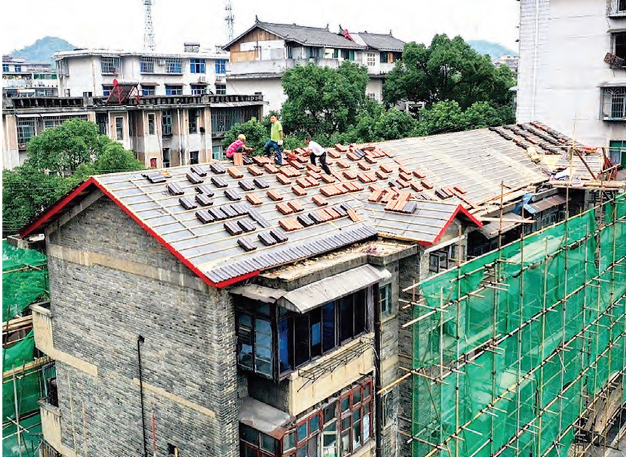
An old residential building in Shuangjiang township, Tongdao Dong autonomous county, Huaihua, central China's Hunan province is being renovated, August, 2022. [People's Daily Online/Li Shangyin]
