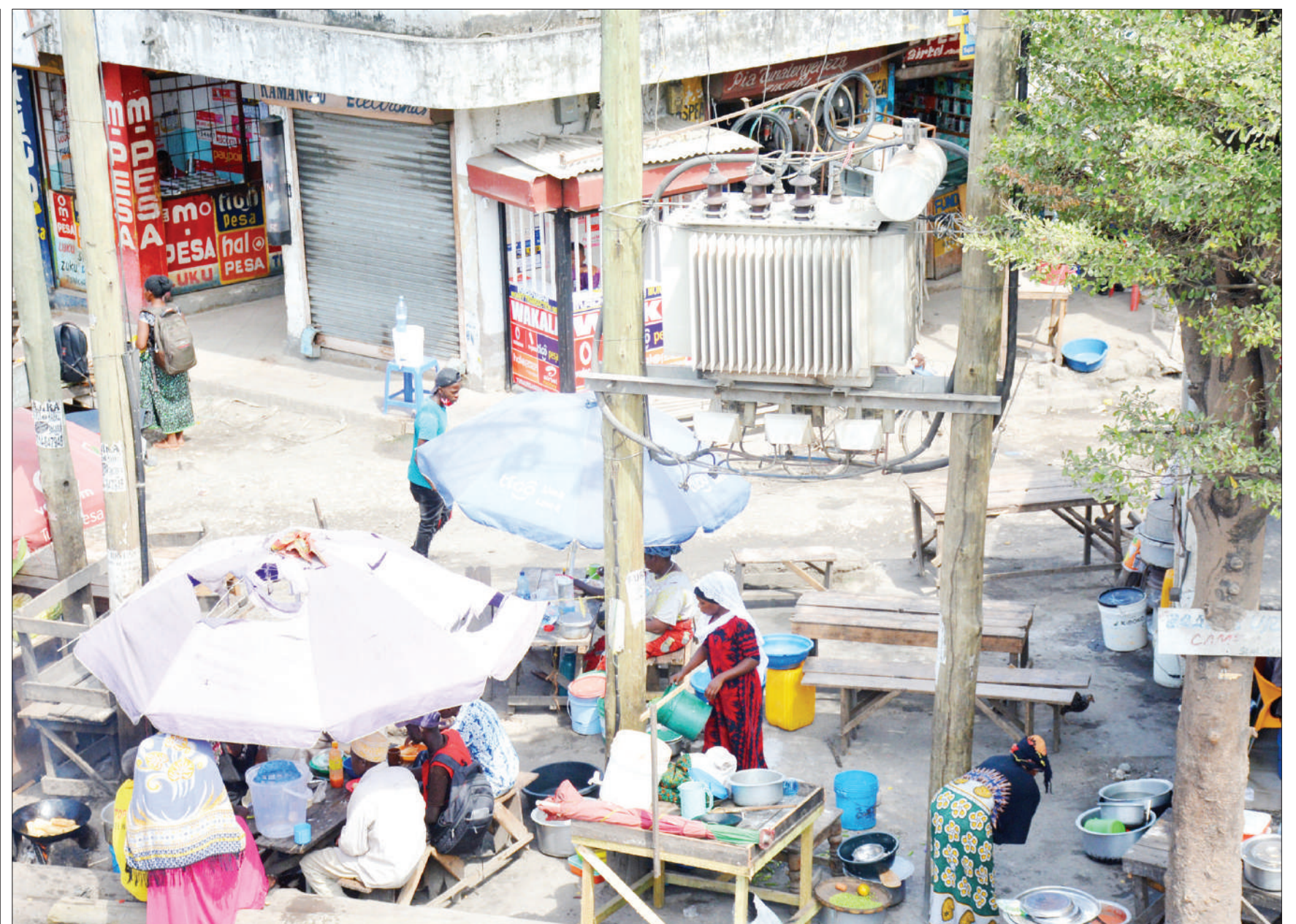
HIGH RISK: Small traders in business right under a transformer and high-tension power lines at Kitunda on the outskirts of Dar es Salaam, as found yesterday - and with each passing day, for quite some time now. Photo: Correspondent Jumanne Juma
