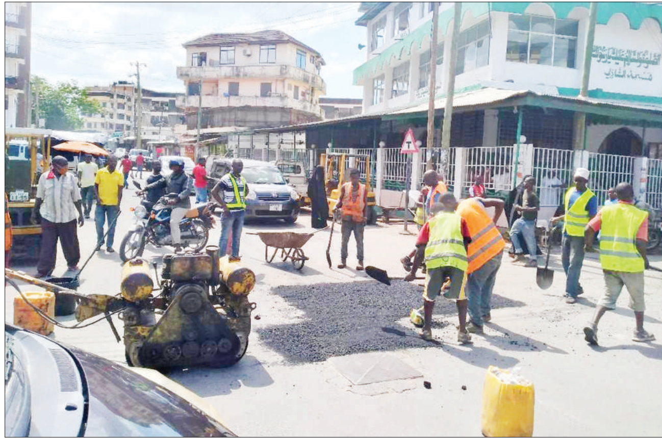
A section of a road near the junction of Dar es Salaam's Sikukuu and Twiga streets undergoes repair yesterday. Photo: Correspondent Joseph Mwendapole
