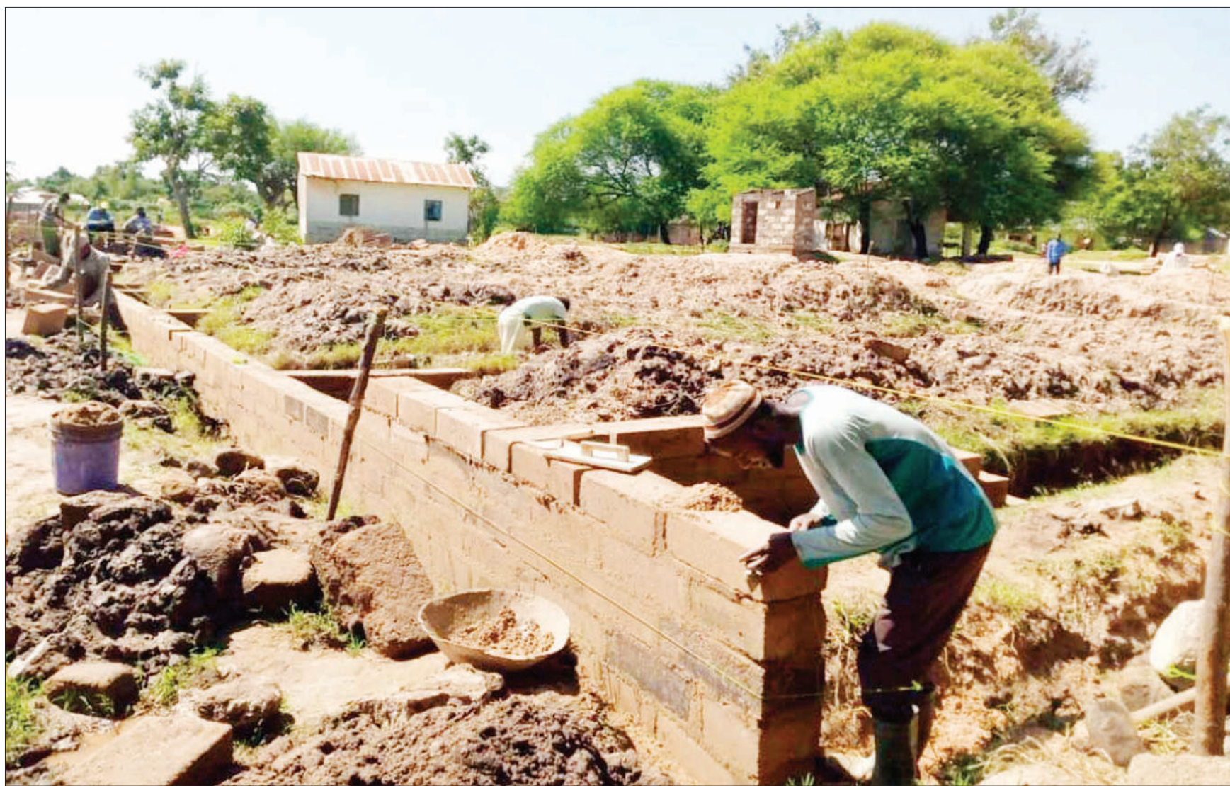
Construction of a maternity and child ward building at Bukima village dispensary in Musoma Rural constituency has begun in earnest, as witnessed earlier this week. Photo: Guardian Correspondent
