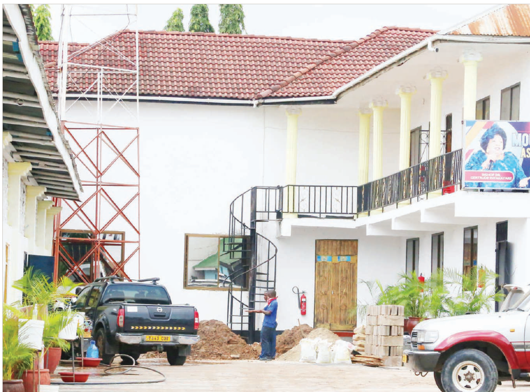
Work on the grave where the long-serving head of the Mikochei B Assemblies of God church, Rev Dr Gertrude Rwakatare, will be buried in Dar es Salaam today under way yesterday. Photo: Selemani Mpochi
