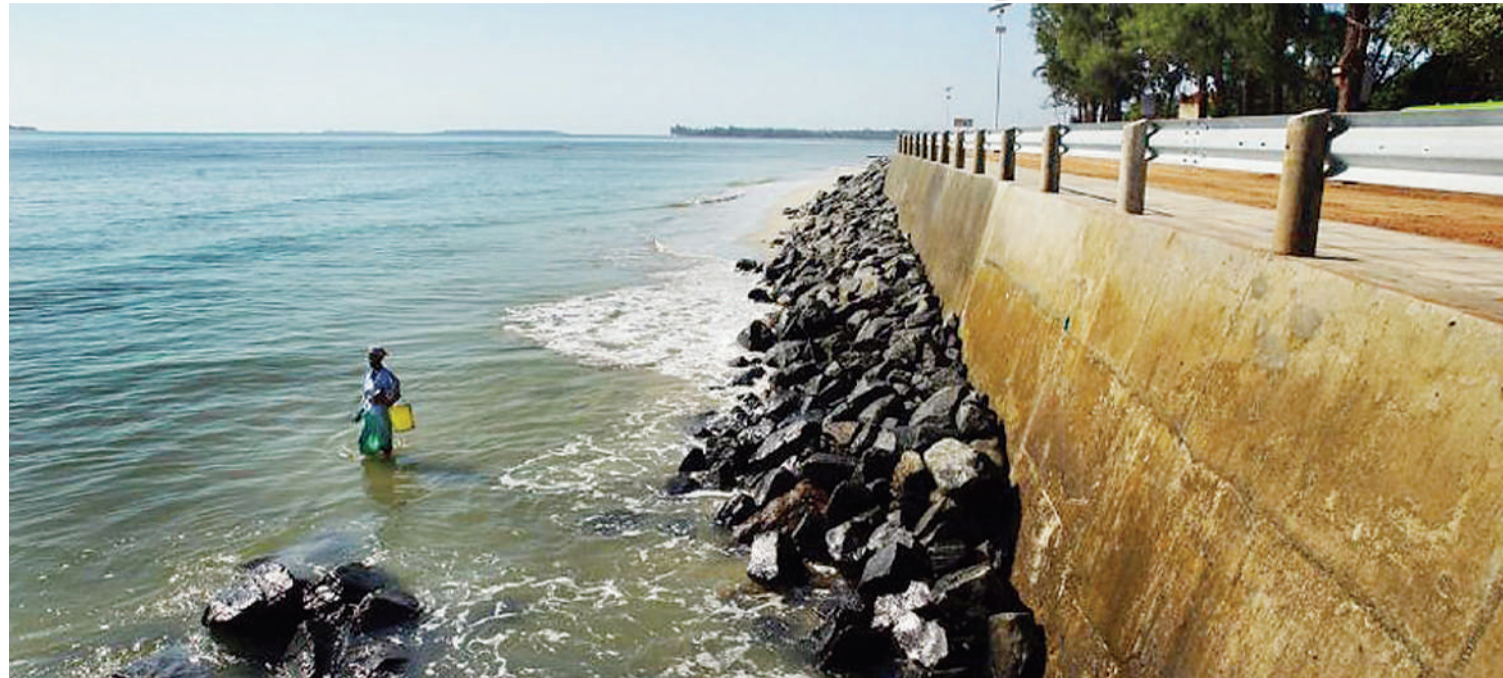
A woman collecting seashells next to the new seawall built along Barack Obama Road in Dar es Salaam to protect the road against rising sea waves.
