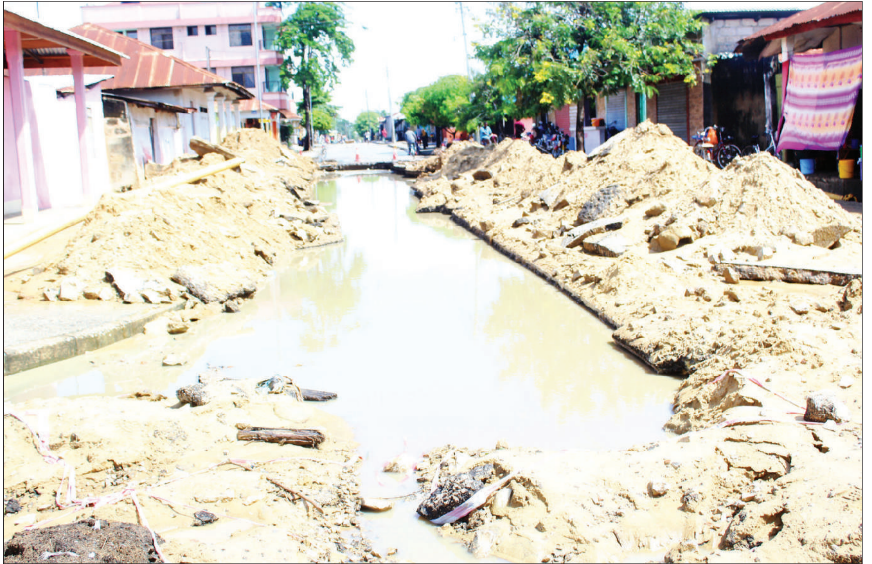
The rehabilitation of this Tanga city street has stalled for quite some time, seriously inconveniencing road users. Correspondent Oscar Kasimiri's roving camera captured this scene yesterday.
