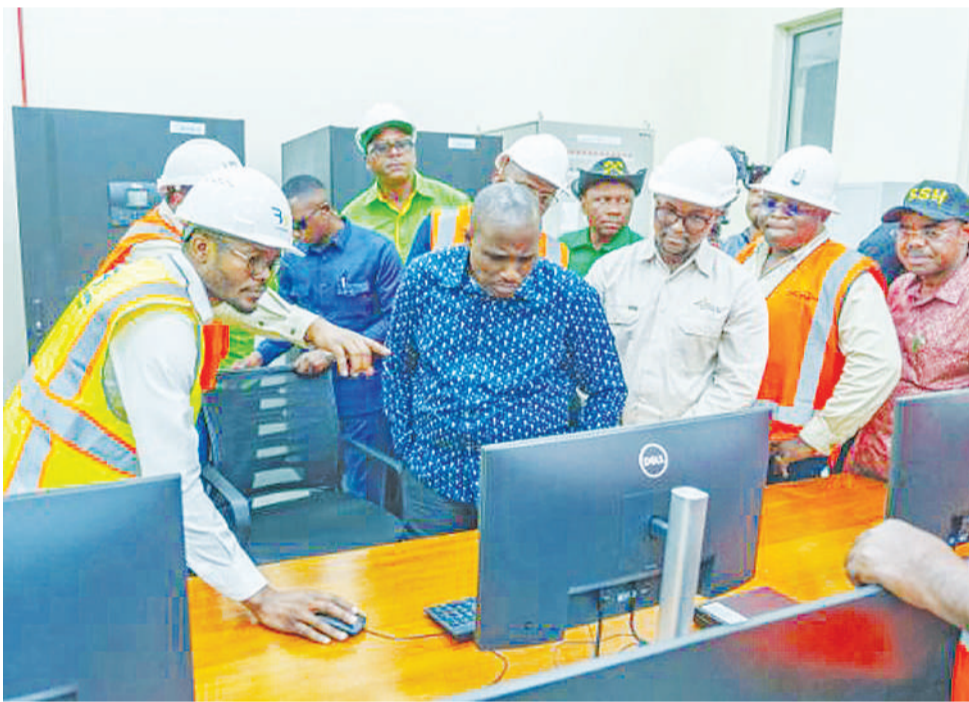
Deputy Prime Minister and Energy minister Dr Doto Mashaka Biteko is briefed on GGML's 33/11KV Substation in the control and switch yard room during the inauguration event. Others are Abrahamu Nzowa - GGML Electrical Engineer 2, Eng. Seif Maftah - GGML Principal Reliability Engineer, Constantine Kanyasu - Geita Urban Constituency MP, and Martin Shigella - Geita's Regional Commissioner. Photo: Guardian Correspondent
