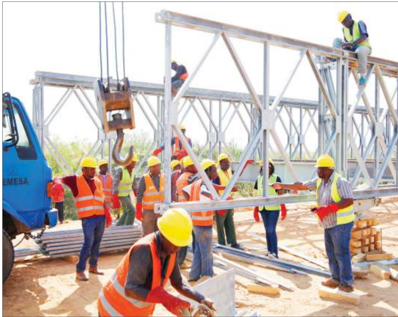
Tanzania Rural and Urban Road Agency (TARURA) engineers and technicians in business at the Mabey Bridge construction site in Melela ward, Kilombero District, yesterday. Photo: Guardian Correspondent
