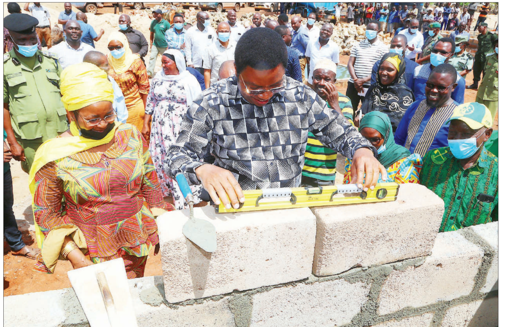
Prime Minister Kassim Majaliwa takes part in the construction of a Mivuleni health centre building in Mchinga ward, Lindi Region, yesterday. Left is Mchinga legislator Salma Kikwete. Photo: PMO
