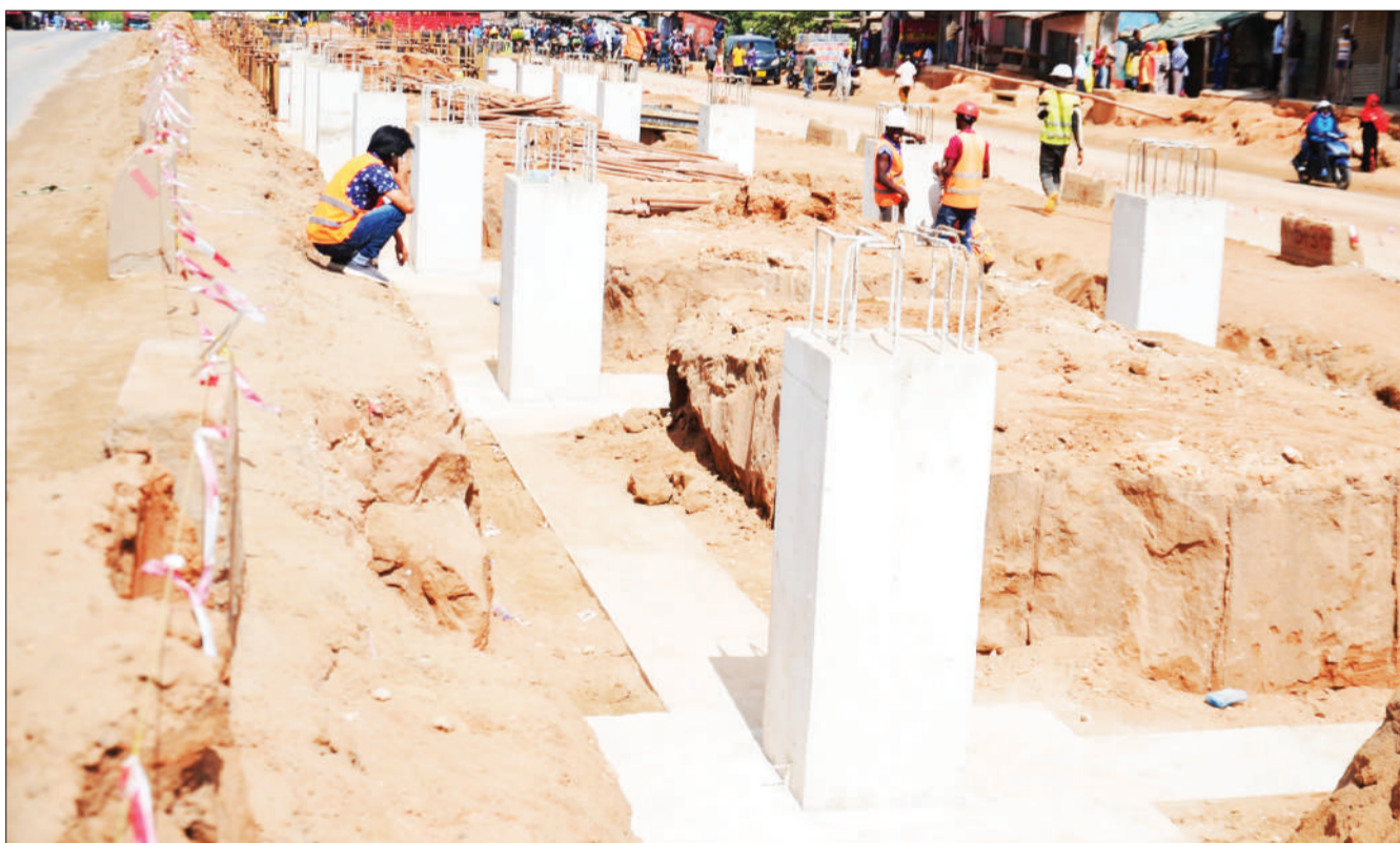
Work on Dar Rapid Transit road infrastructure from Mbagala to downtown Dar es Salaam in progress along the Mtoni Mtongani stretch of Kilwa Road yesterday. Photo: Correspondent Jumanne Juma
