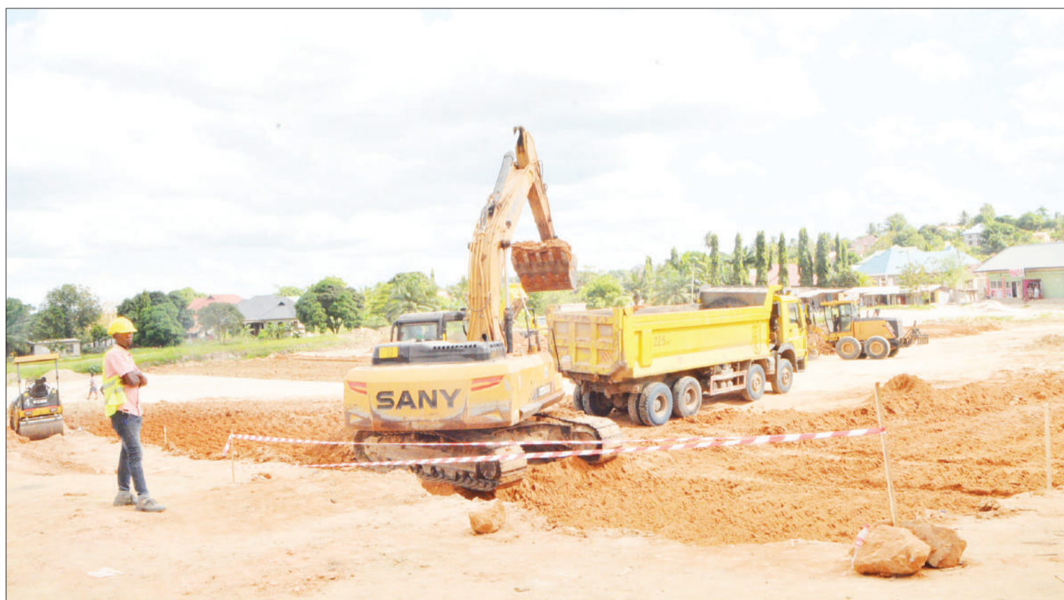
A scene at one of the sites at Kinyerezi in suburban Dar es Salaam where China Railway Seventh Group Company Limited is soon to build a commuter bus stand, as captured yesterday. Photo: Correspondent Miraji Msala
