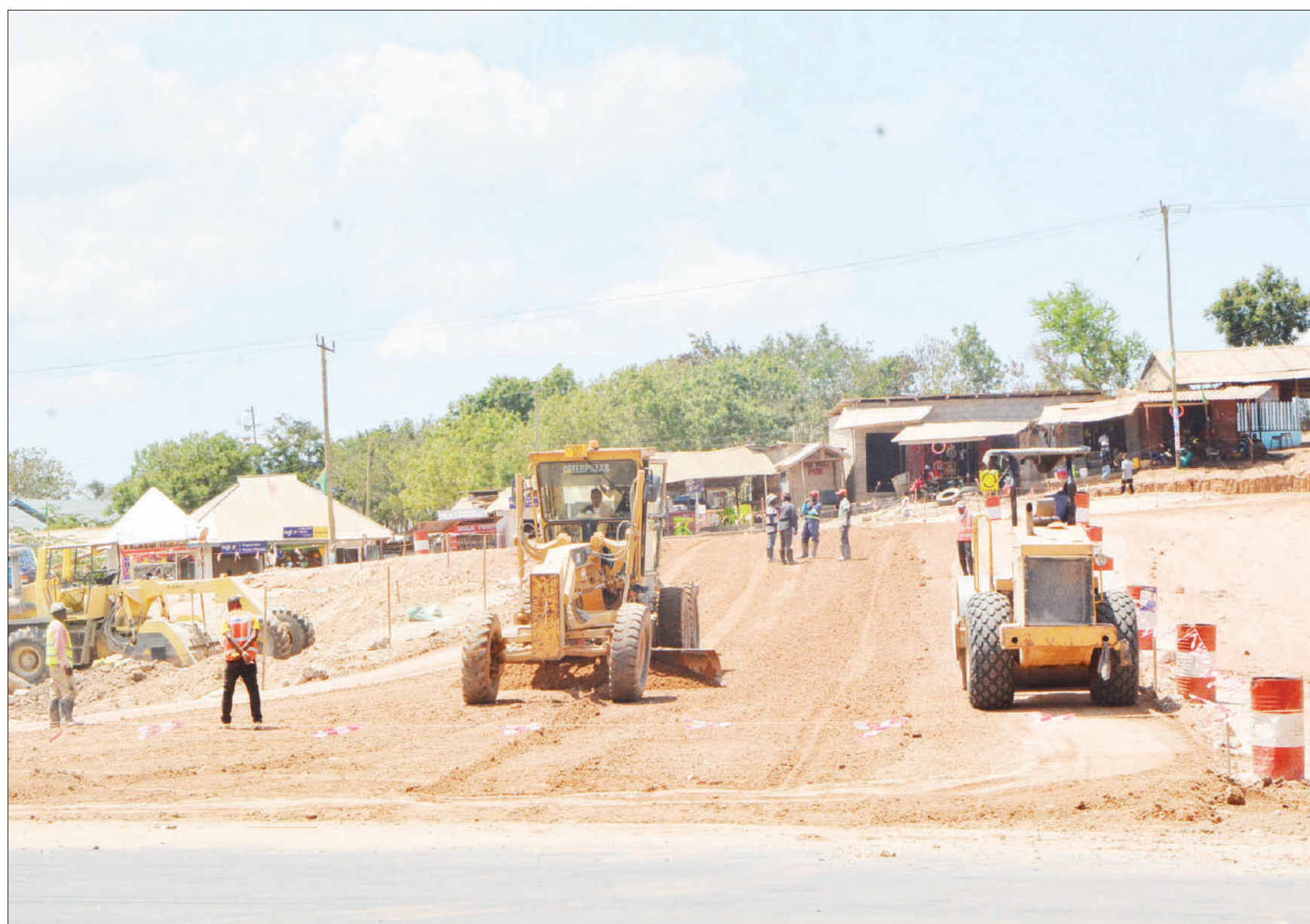
Road construction under way in Dar es Salaam's Kibamba suburb yesterday. Photo: Correspondent Miraji Msala
