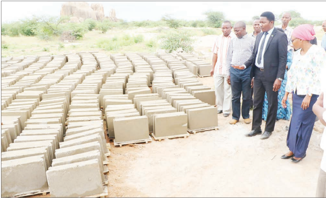
Minister of State in the President's Office Regional Administration and Local Government Selemani Jafo (3rd L) inspects the ongoing construction of infrastructure in Bahi district, Dodoma region yesterday. Photo: Correspondent Paul Mabeja
