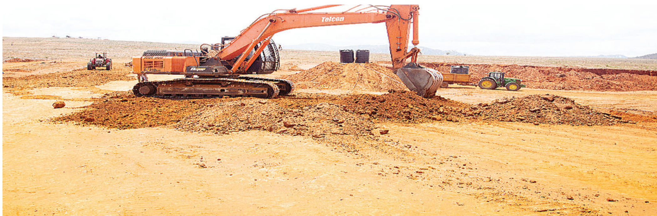
Construction of an irrigation dam is in top gear at Farm for the Future commercial farm in Iringa where a 250-hectare investment in production of seed maize and macadamia is expected to kick off from October 2022. Photo: Guardian Correspondent.
