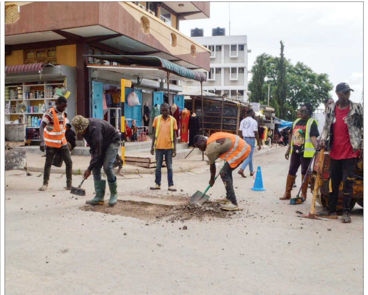
Repair of a section of Iringa municipality's Soko Kuu in progress, as found yesterday. It's periodic maintenance forming part of a Tanzania Rural and Urban Roads Agency (TARURA) project. Photo: Correspondent Friday Simbaya
