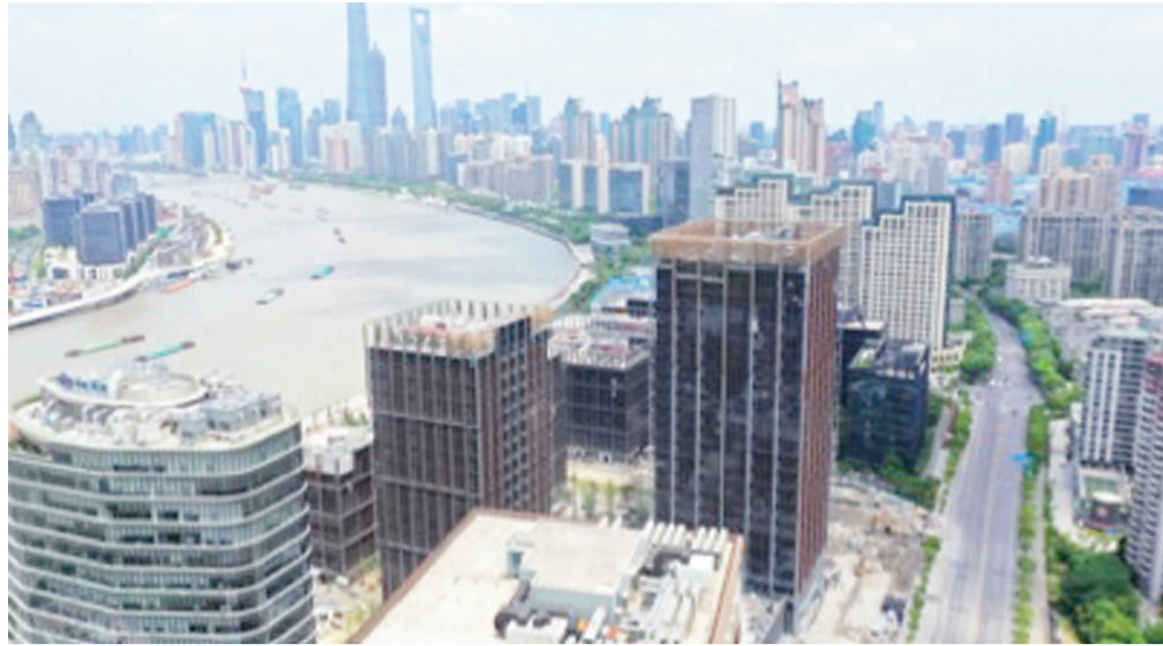
An aerial photo shows the construction site of an office building project at the Binjiang Avenue in Pudong, Shanghai. The project represents the largest commercial building complex along Binjiang Avenue. File photo
