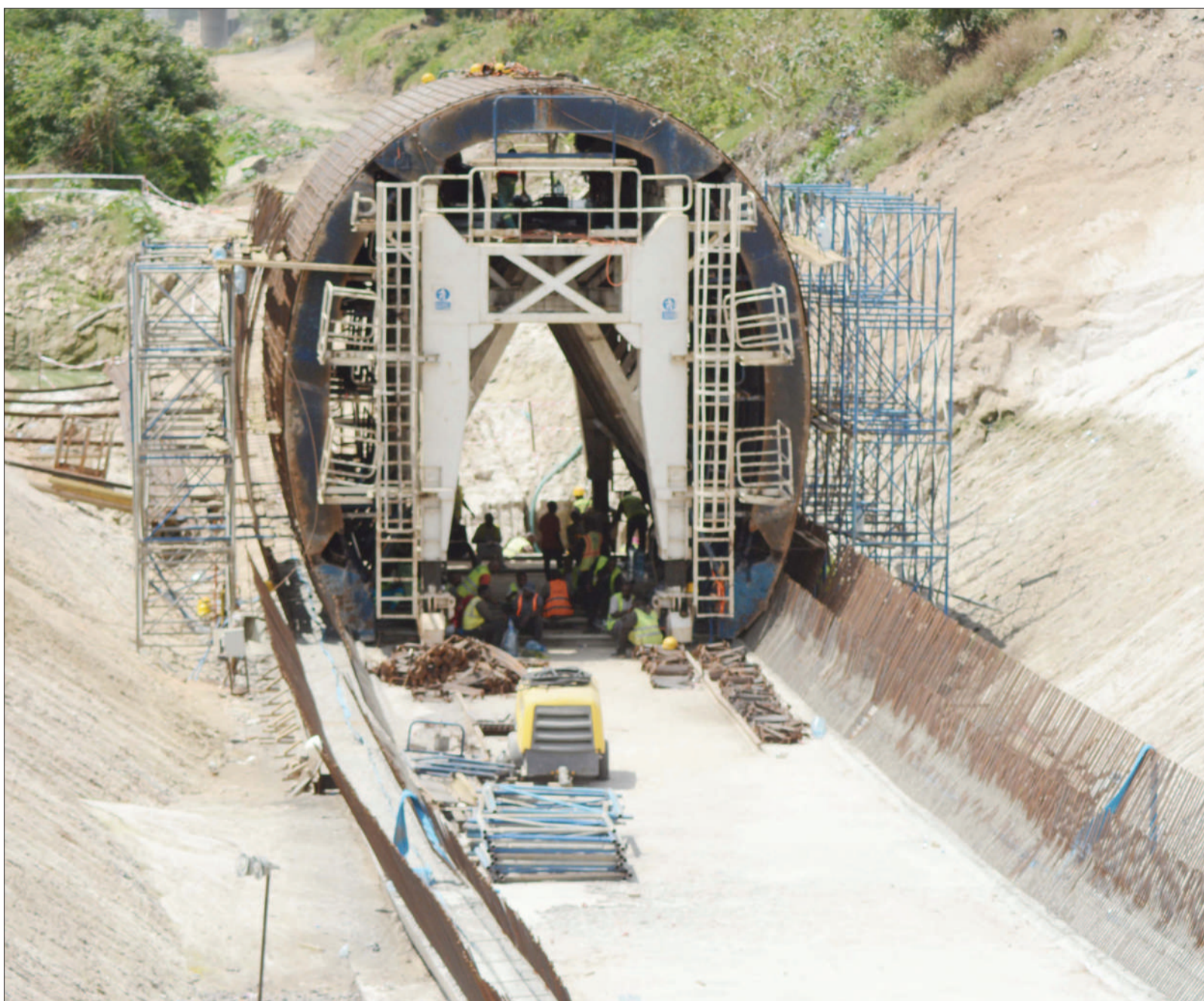
Rehabilitation gets well under way yesterday on a strategic bridge along Dar es Salaam's Darajani Chang'ombe section of the Central Railway Line. Photo: Correspondent Jumanne Juma
