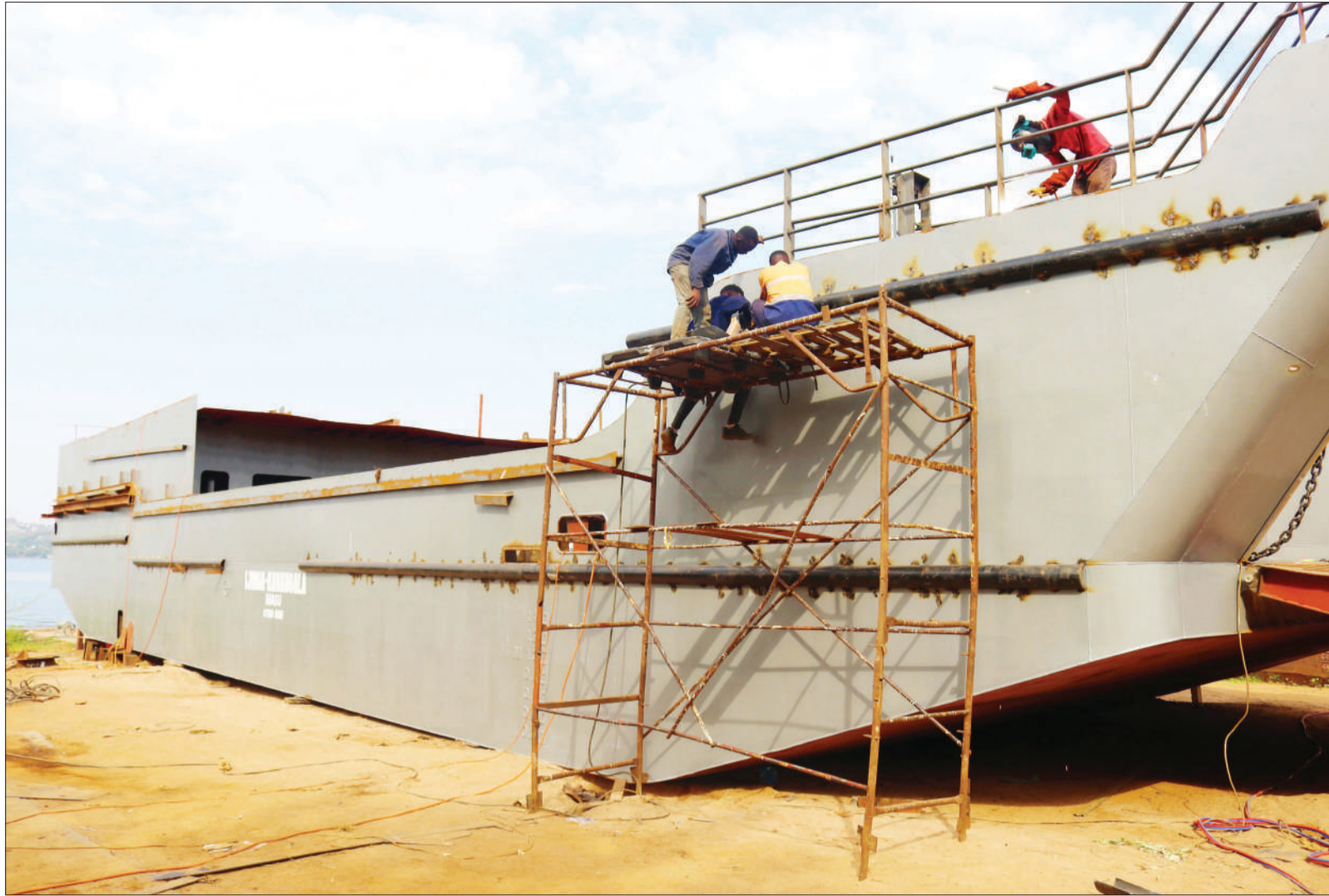
Construction of a 5.2bn/- ferry meant to serve the Ijinga-Kahangara route in Magu District well under way at the Songoro Marine garage at Ilelela in Mwanza Region, as witnessed yesterday. It will have capacity for 200 passengers and ten motor vehicles weighing a combined 100 tonnes. Photo: Guardian Correspondent
